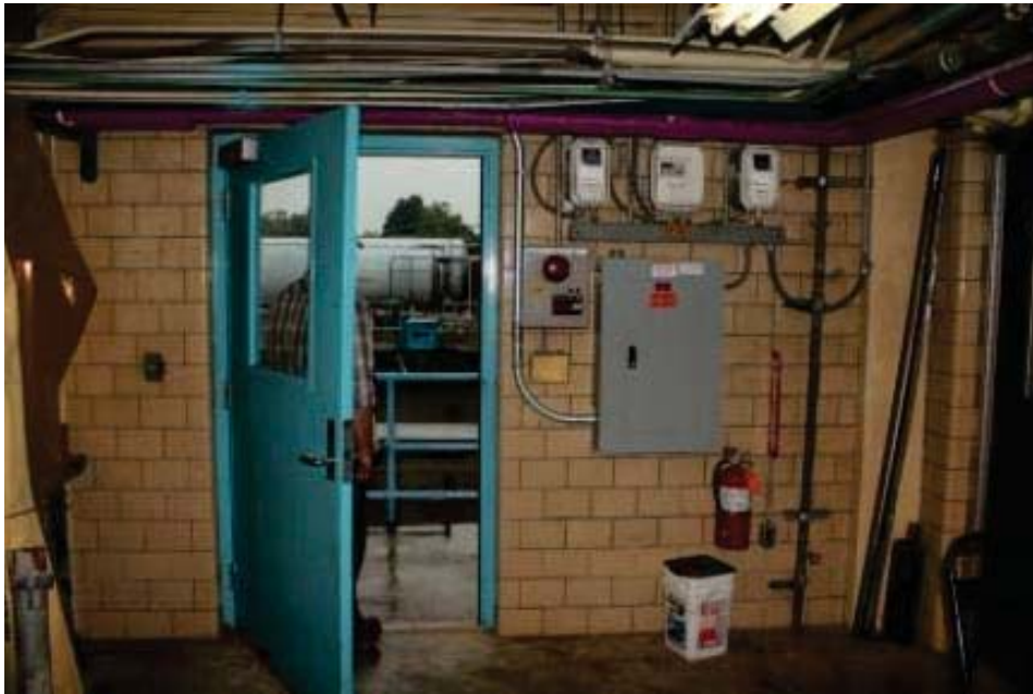
Flocculation Basin No. 3 Electrical/Control
