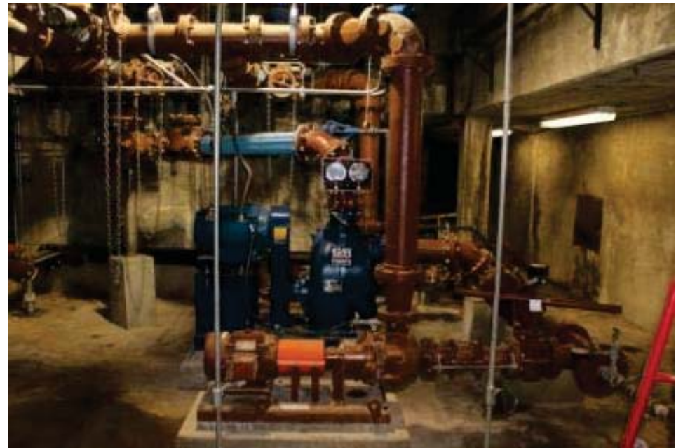
Sludge Pumps 3A & 3B, Drain Pump 2 and 6-inch Control Valves
