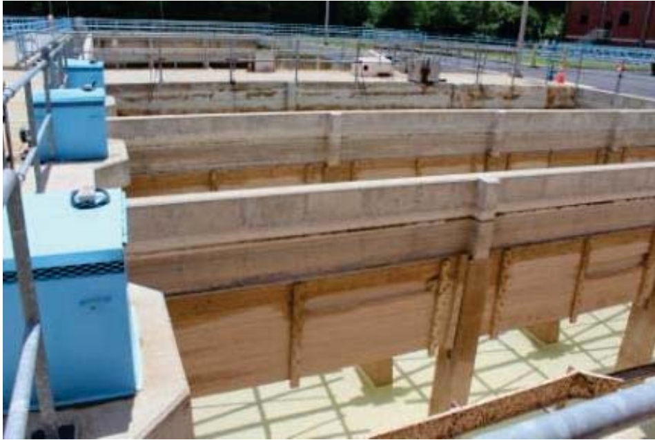
Basin No. 2 Flocculator Drives and Baffles
