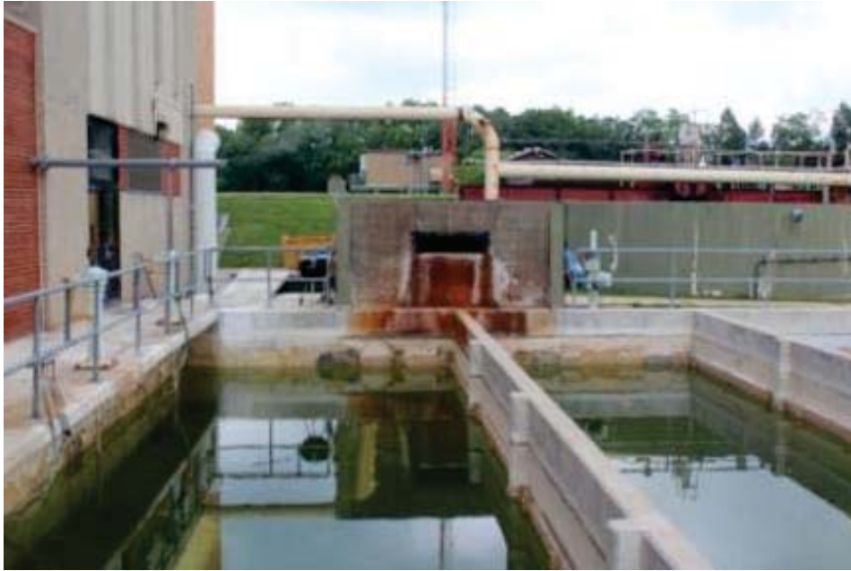
Well Water Influent Chamber/Overflow
