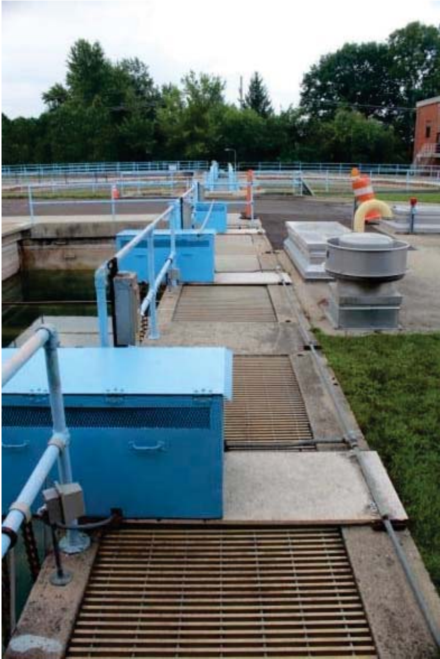
Flocculation Basin No. 3 Flocculator Drives
