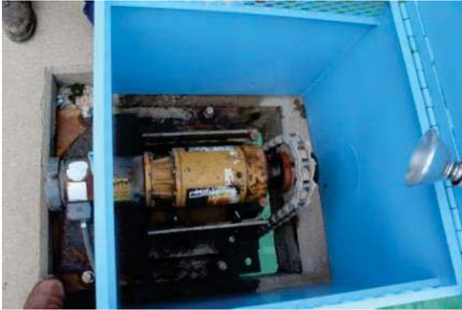
Basin No. 1 Flocculator Drive, Chain, and Upper Sprocket
