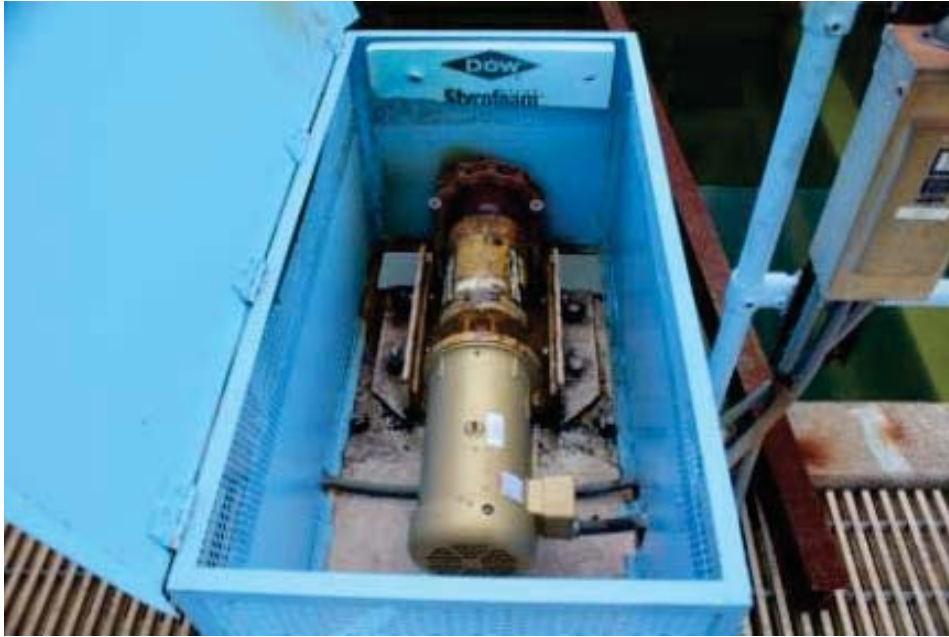
Flocculation Basin No. 3 Flocculator Drive and Upper Sprocket
