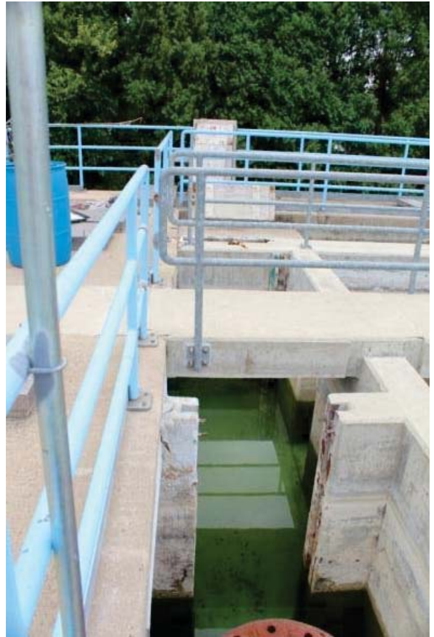
Basin Nos. 1 & 2 Effluent Stop Log Frame
