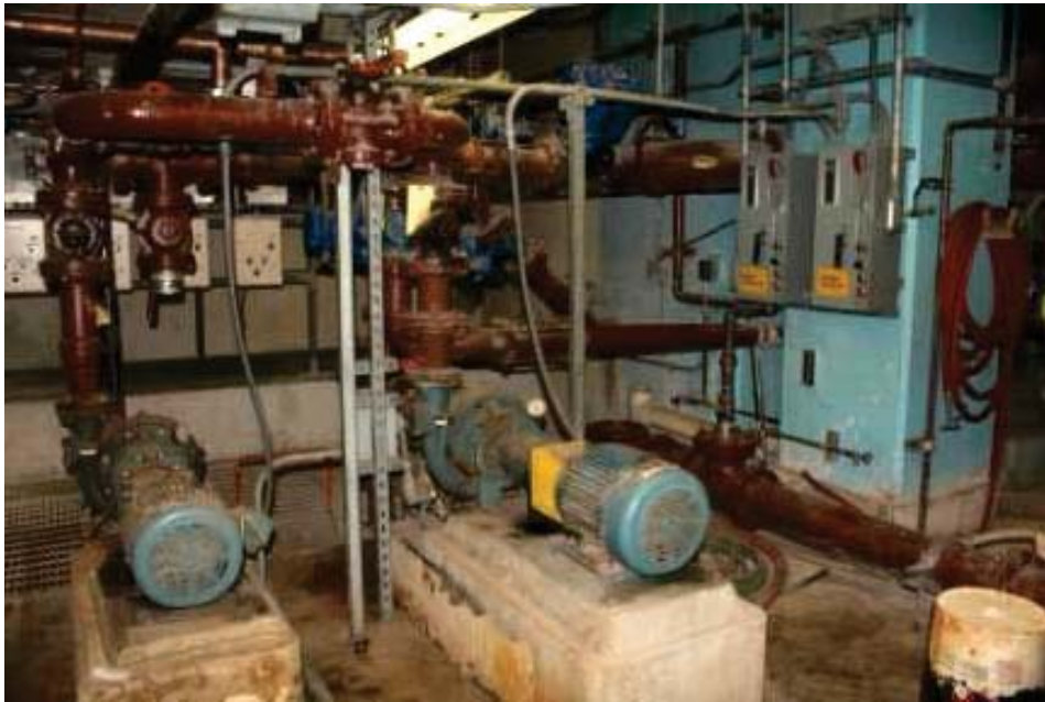
Sludge Pumps 1 & 2, 4-inch Sludge and Control Valves (Basin 1 & 2)
