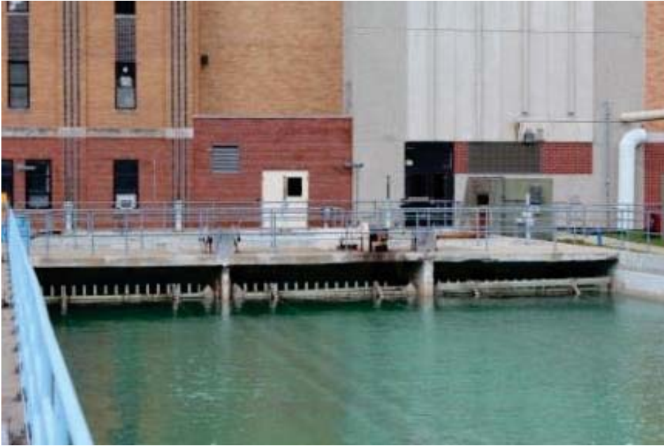
Basin No. 1 Sludge Collection Drive and Upper Sprockets
