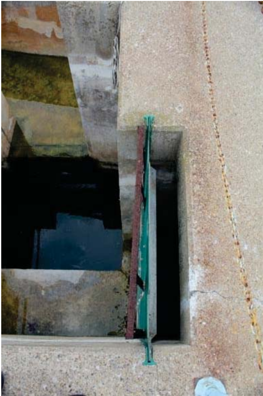
Basin No. 3 North Effluent Structure and Slide Plate
