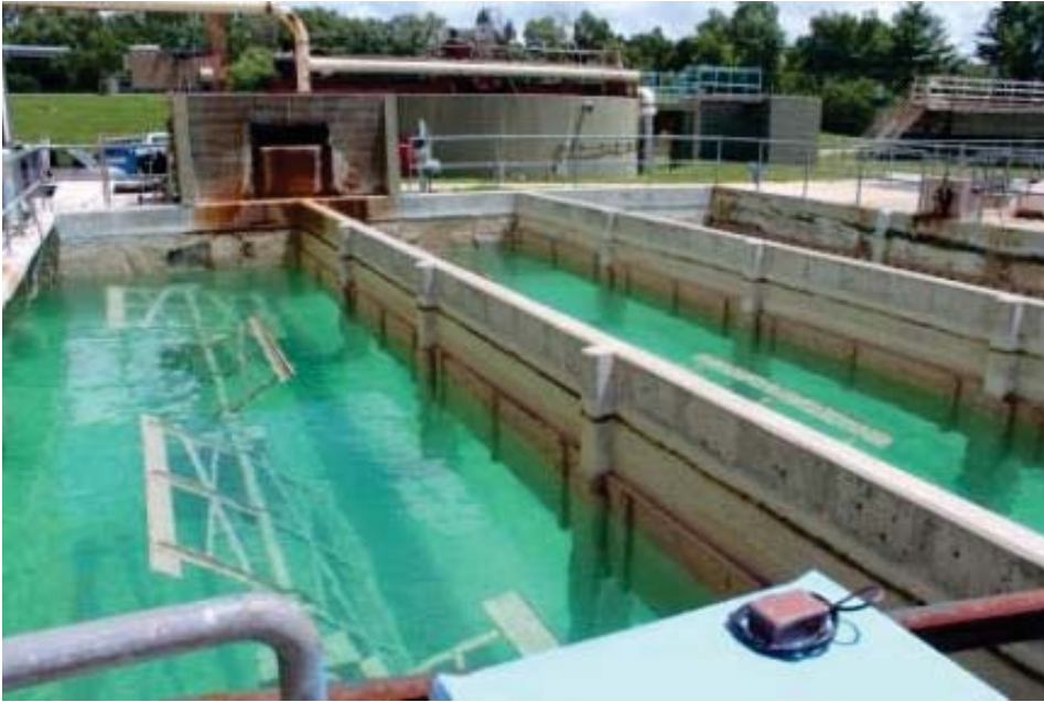
Basin No. 1 Stage 1 & 2 Flocculators and Baffles
