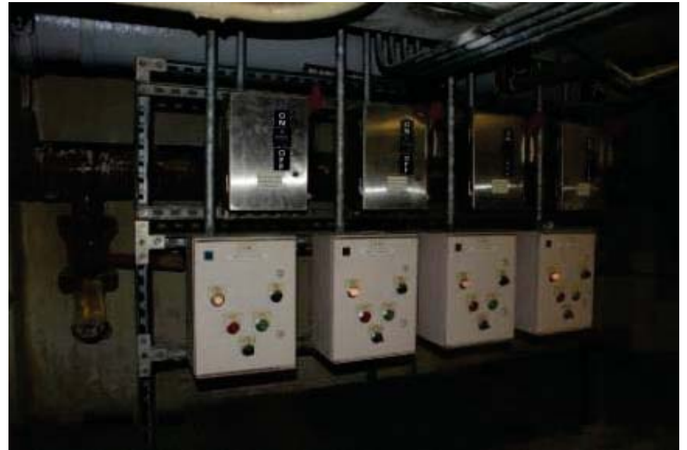
Motorized Sludge Valve Electrical/Control (Basin 1 & 2)
