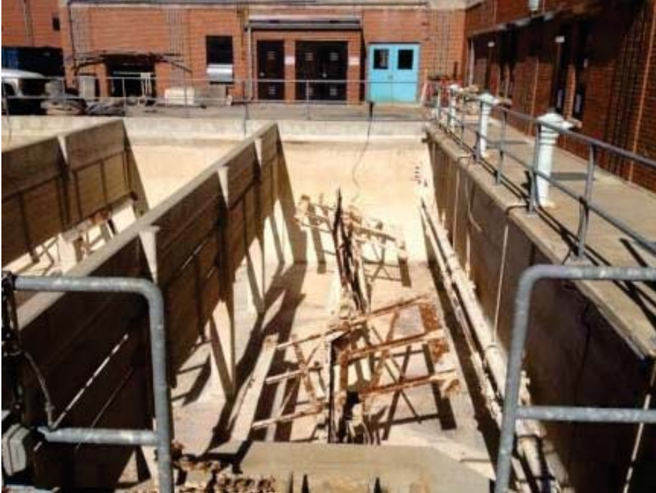
Basin No. 2 Stage 1 Flocculator
