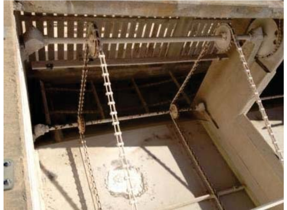
Basin No. 2 Cross Collector and Sludge Collection Chain & Sprockets
