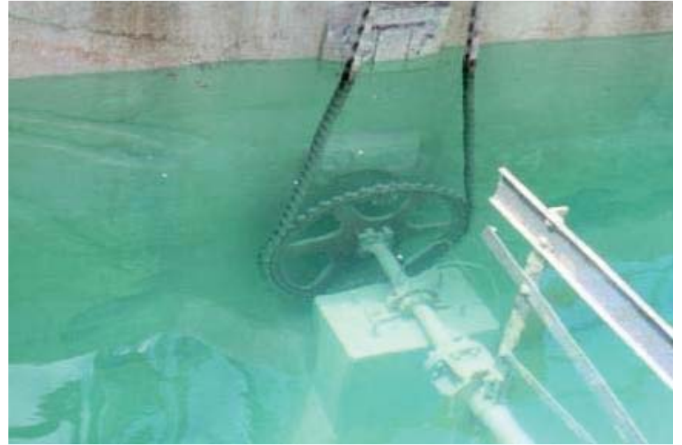
Basin No. 1 Flocculator Chain & Lower Sprocket
