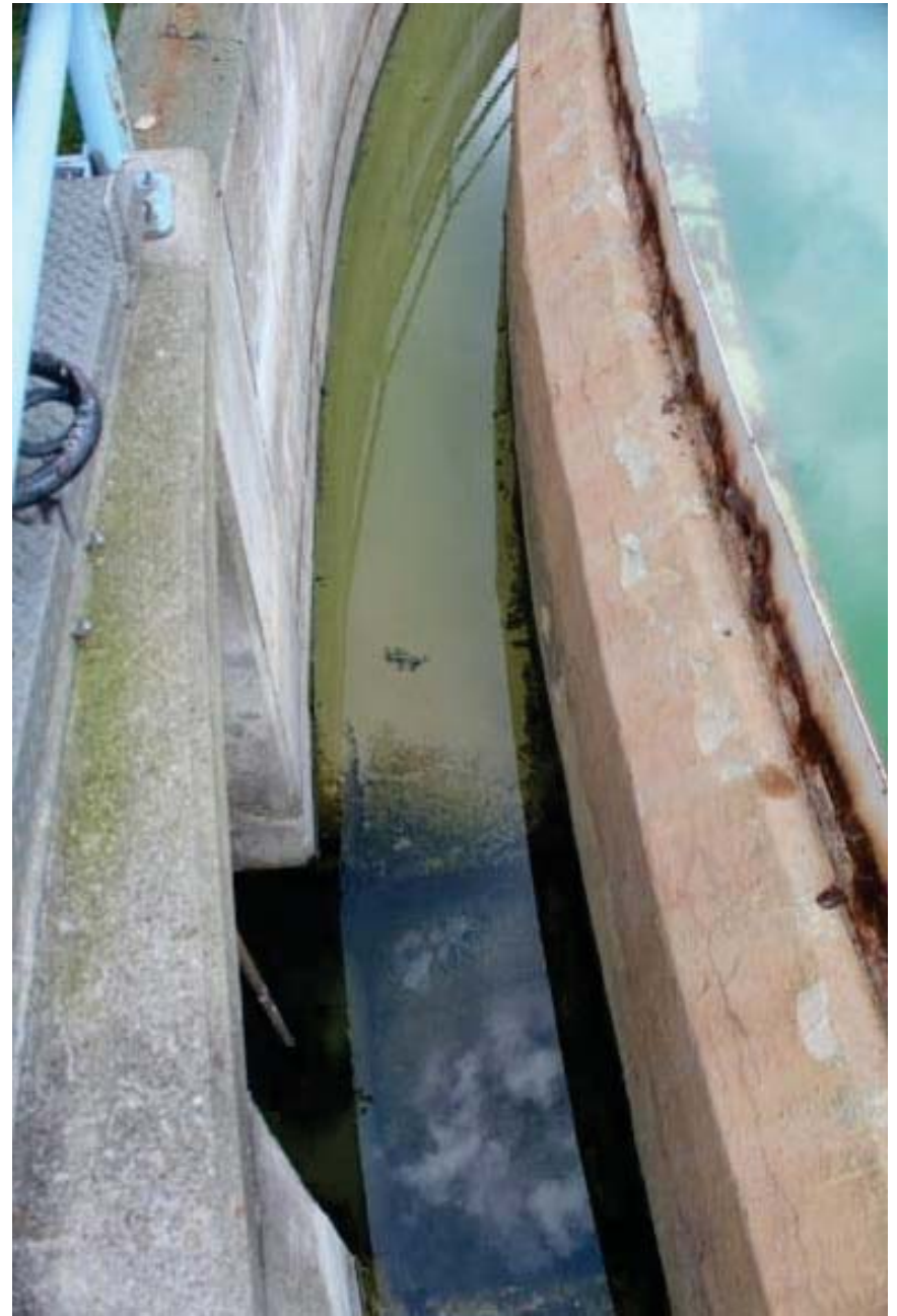
Basin No. 3 Effluent Weir, South Effluent Channel, and Effluent Mud Valve
