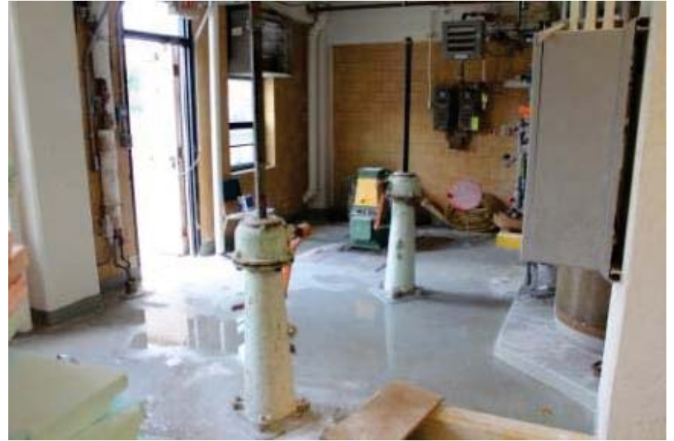
Basin 1 & 2 Influent Isolation Gate Nos. 1 & 2 Actuators
