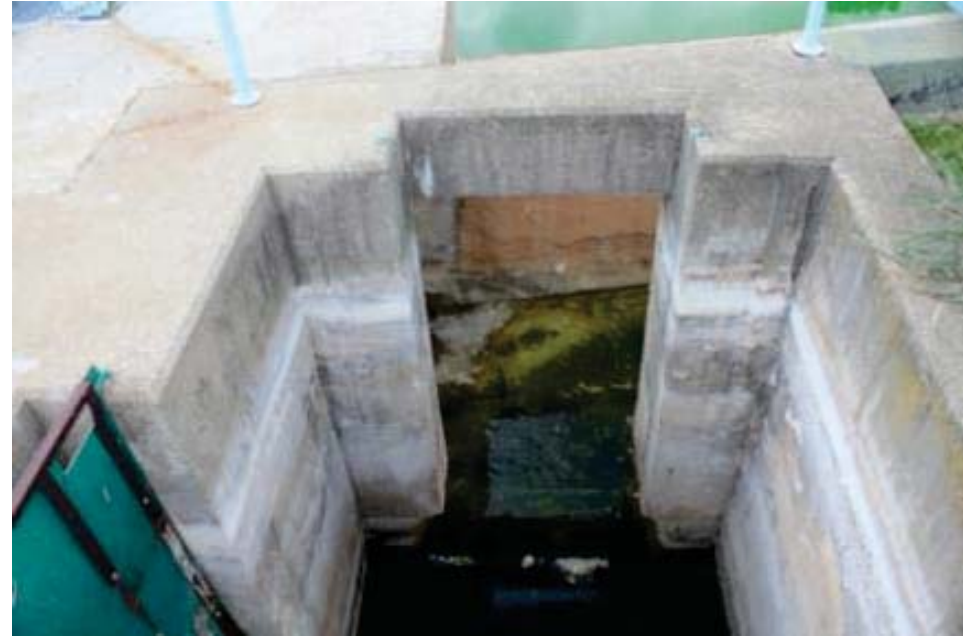
Basin No. 3 North Effluent Structure, Slide Plate, and Slide Plate Frame
