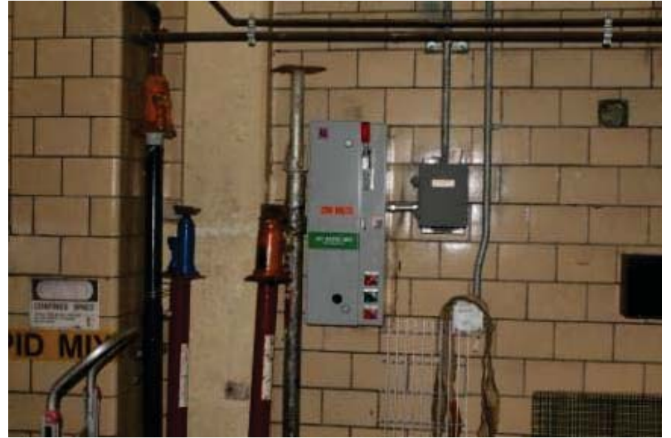
Rapid Mix 3 Electrical/Control
