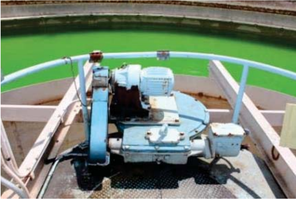
Basin No. 3 Sludge Collection Drive
