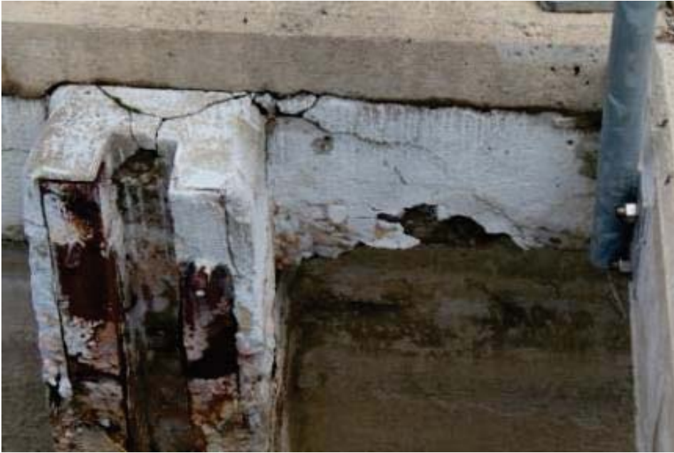
Basin Nos. 1 & 2 Effluent Stop Log Frame
