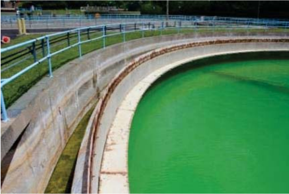
Basin No. 3 Peripheral Wall Baffle, Effluent Weir, and Effluent Channel
