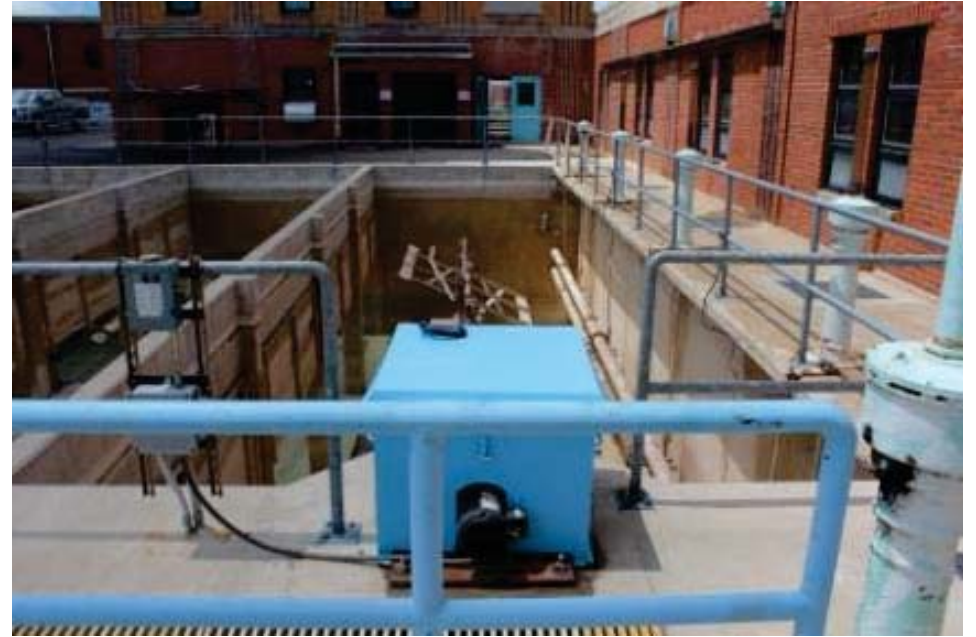
Basin 2 Influent Distribution Gate Actuators and Stage 1 Flocculator Drive
