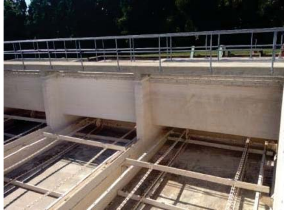
Basin 2 Sludge Collection Equipment and Effluent Weirs
