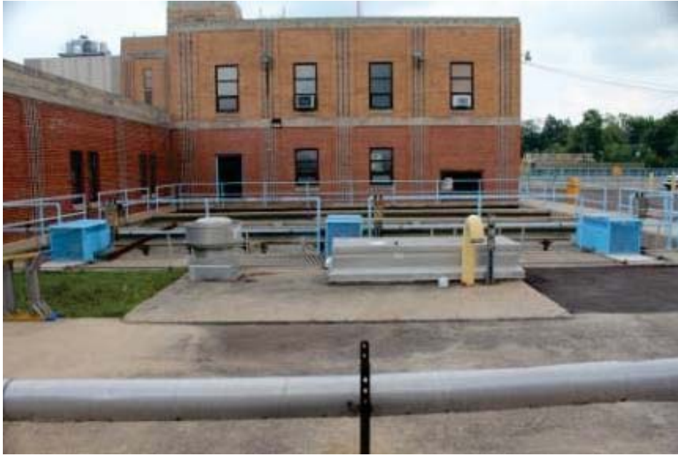
Flocculation Basin No. 3 Flocculator Drives
