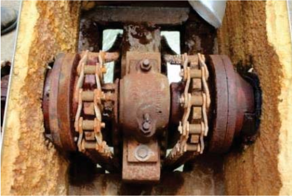
Basin No. 2 Sludge Collection Chain and Upper Sprocket
