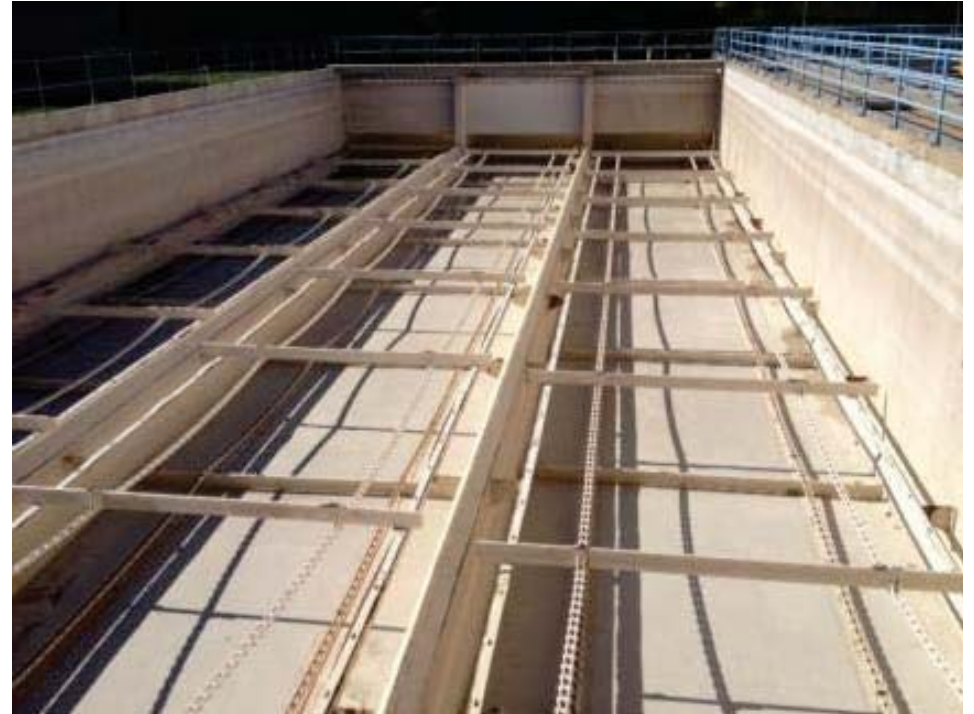
Basin No. 1 Sludge Collection Equipment
