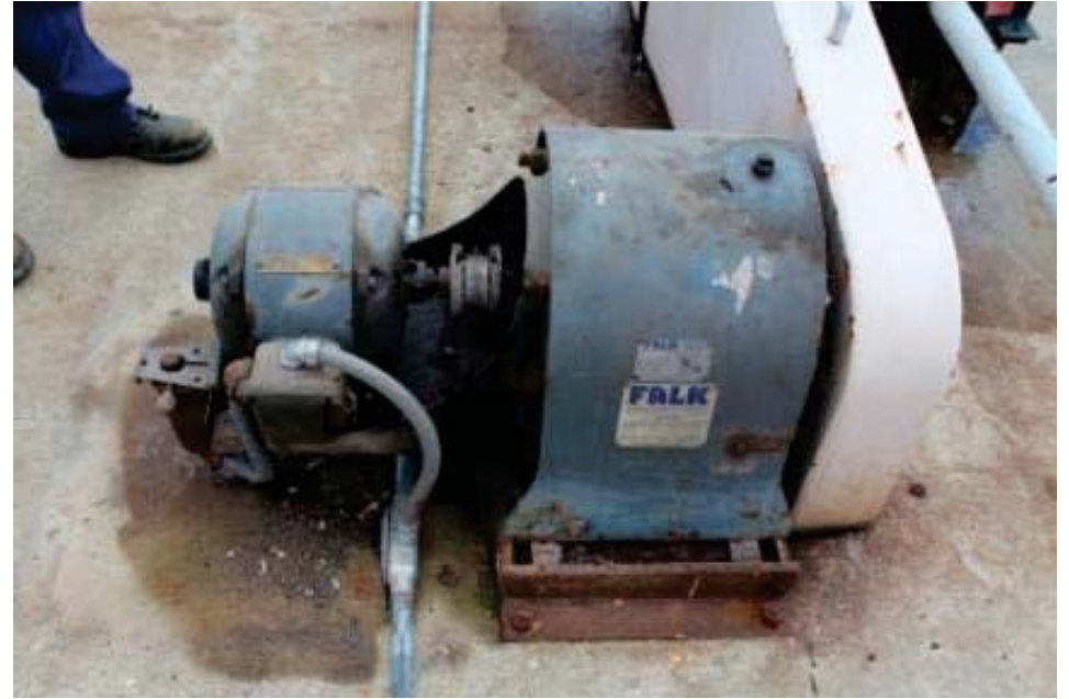
Basin No. 2 Sludge Collection Drive
