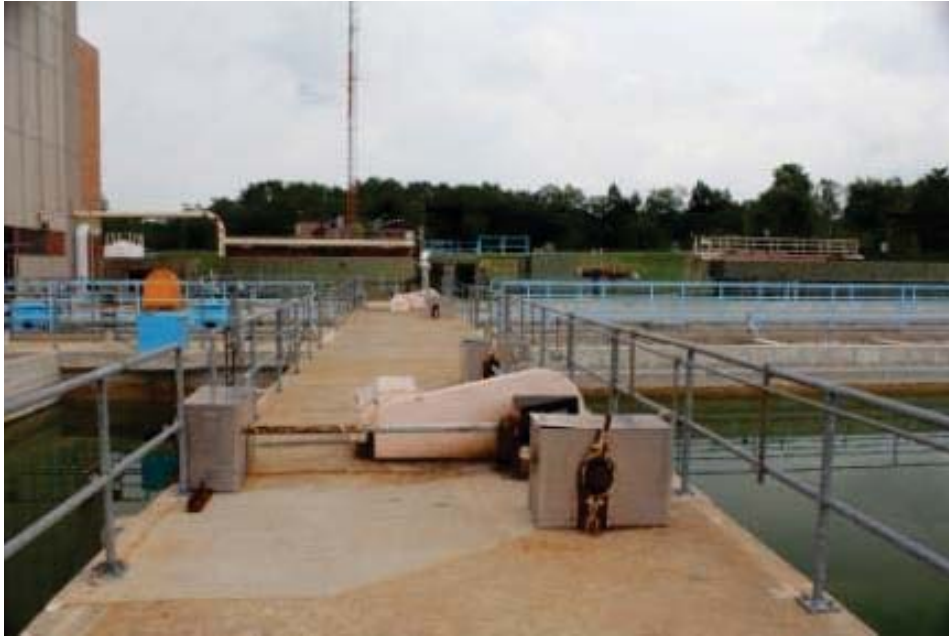
Basin No. 2 Sludge Collection Drive
