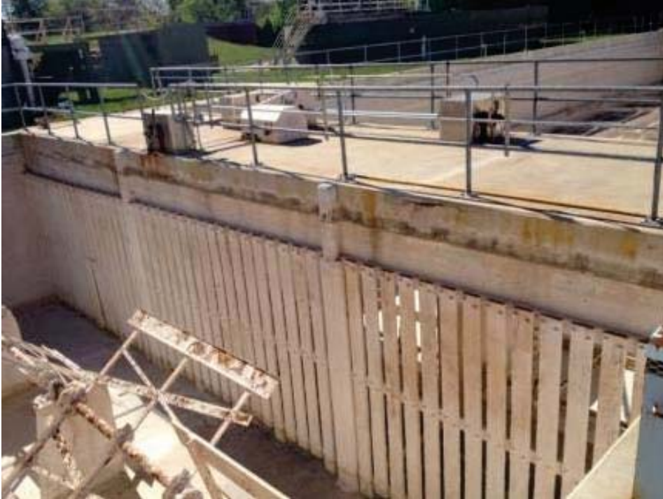
Basin 1 Stage 3 Flocculator and Baffle Wall
