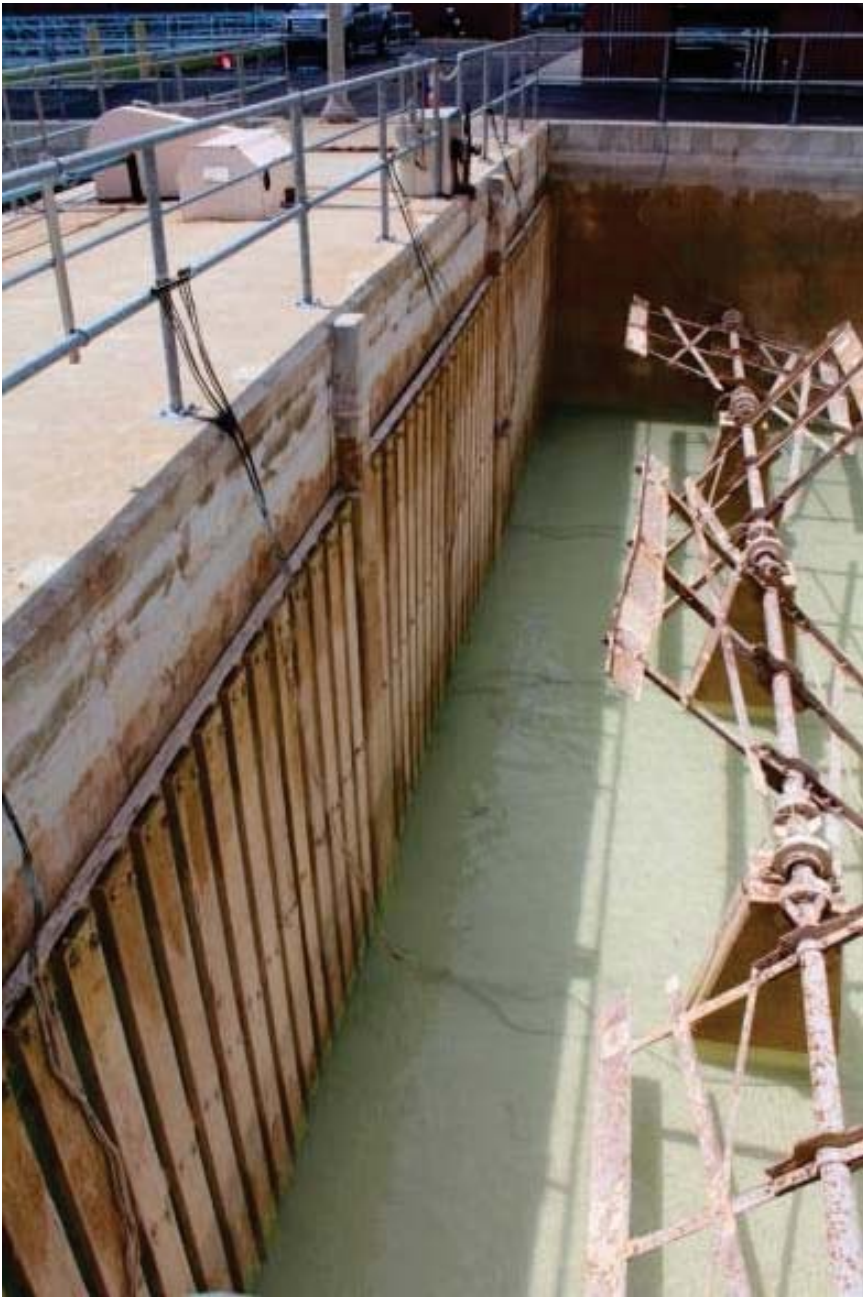
Basin No. 2 Stage 3 Flocculator and Baffle Wall
