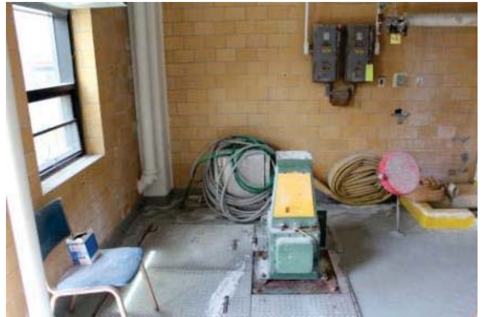
Rapid Mix No. 2 Drive and Rapid Mix 1 & 2 Electrical/Control
