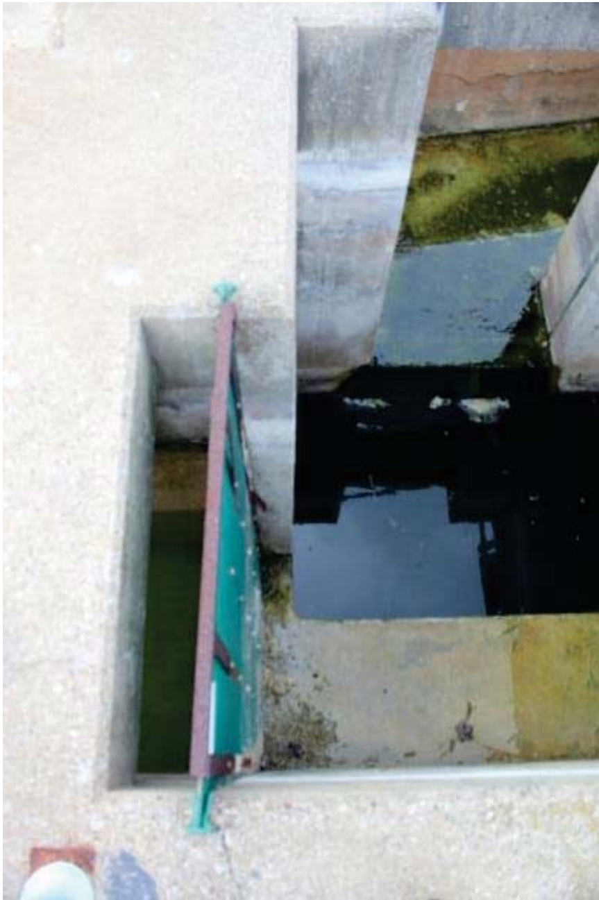
Basin No. 3 North Effluent Structure, Slide Plate, and Slide Plate Frame
