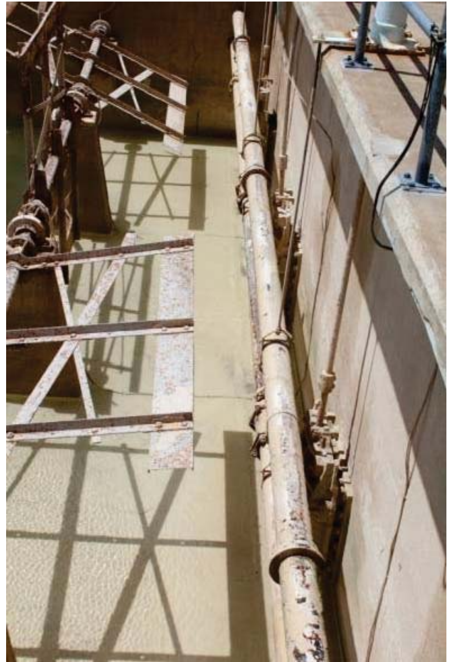
Basin No. 2 Influent Distribution Gates and Sludge Piping
