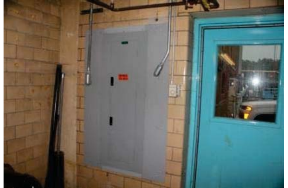
Basin Nos. 1 & 2 Sludge Collection Electrical/Control
