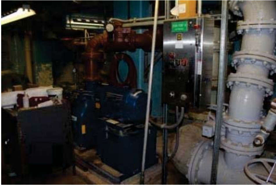
Drain Pump No. 1 and Electrical/Control
