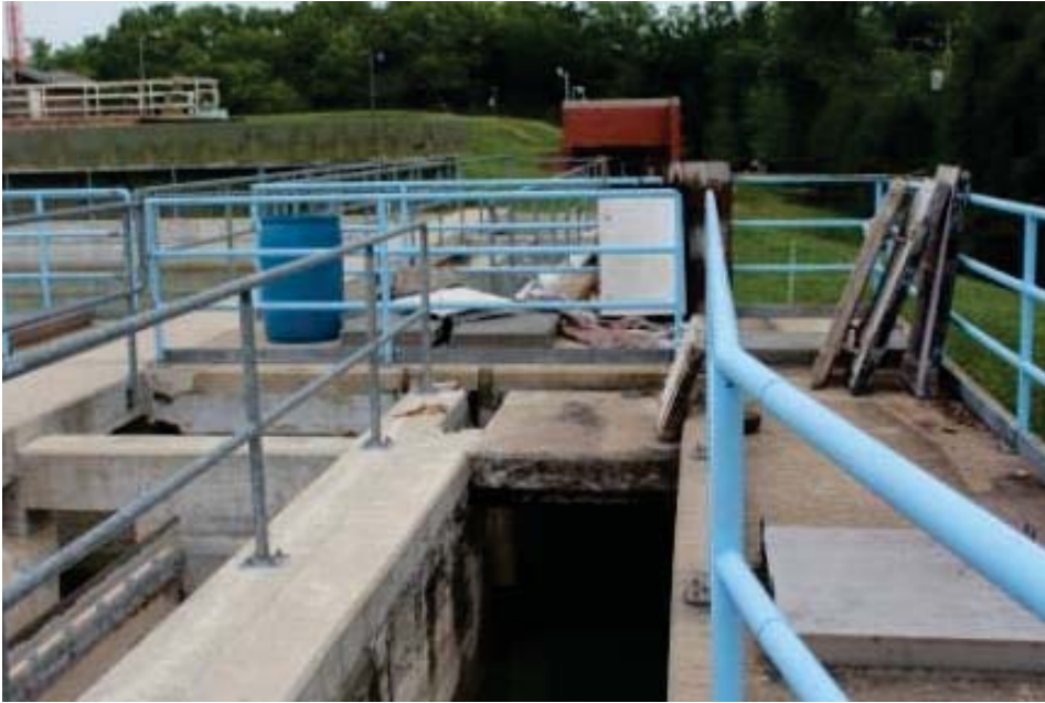
Basin Nos. 1 & 2 Effluent Stop Logs
