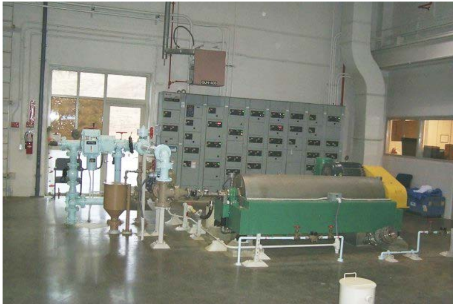
Figure TM4-5: Installed Centrifuge
