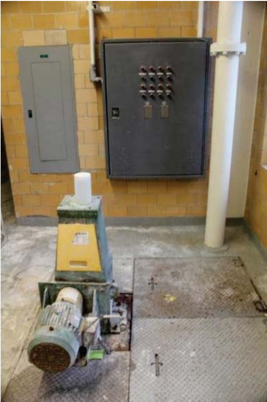
Rapid Mix No. 1 Drive and Basin Nos. 1 & 2 Flocculator Electrical/Control
