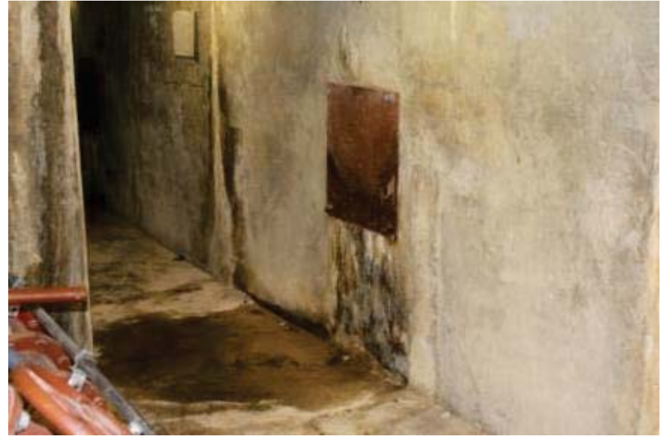
Piping Gallery Wall
