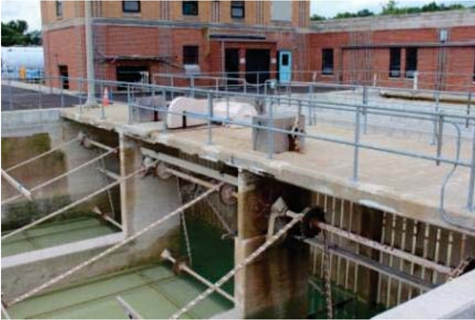
Basin No. 2 Sludge Collection Drive and Equipment
