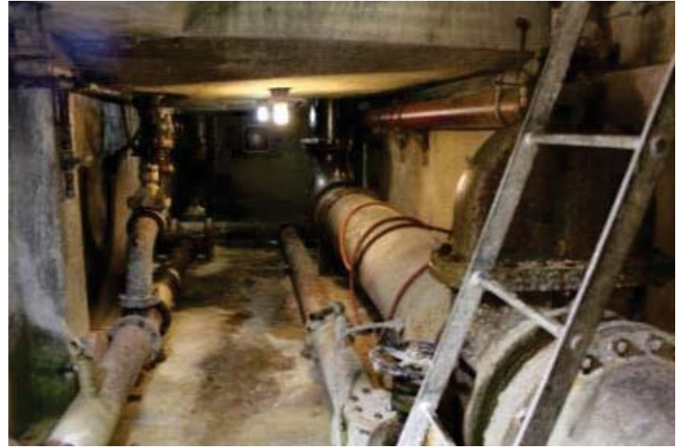
24-inch Raw Influent to Rapid Mix 1 & 2, 8-inch Sludge (Basin 1 & 2)
