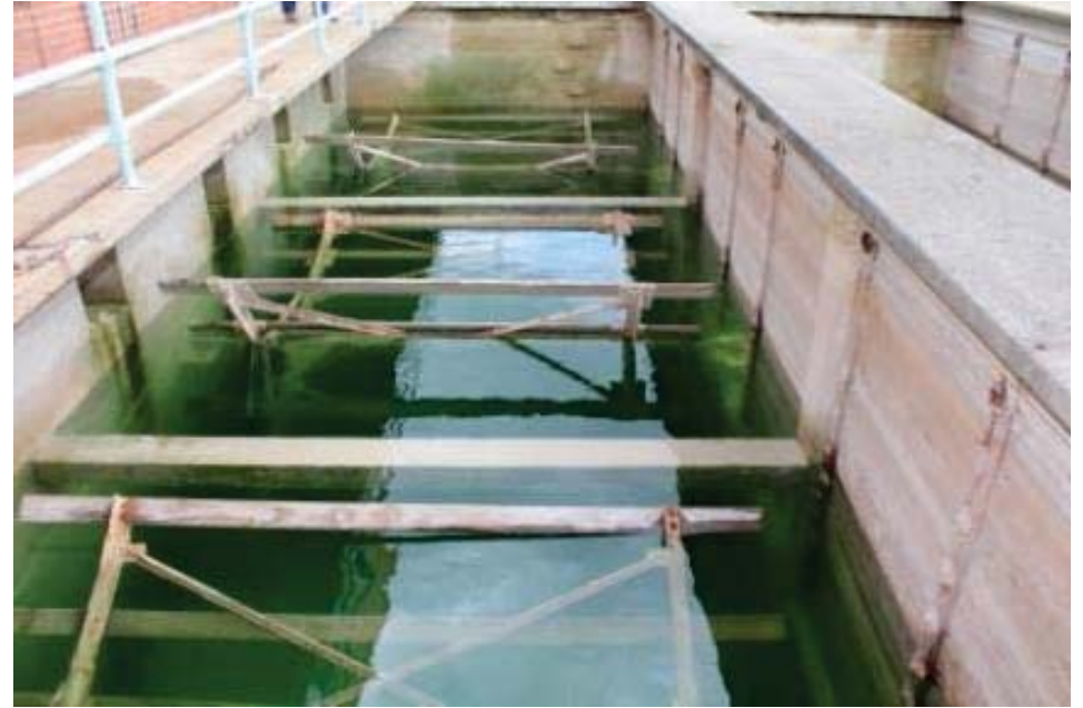
Flocculation Basin No. 3 Stage 1 and Baffle Wall
