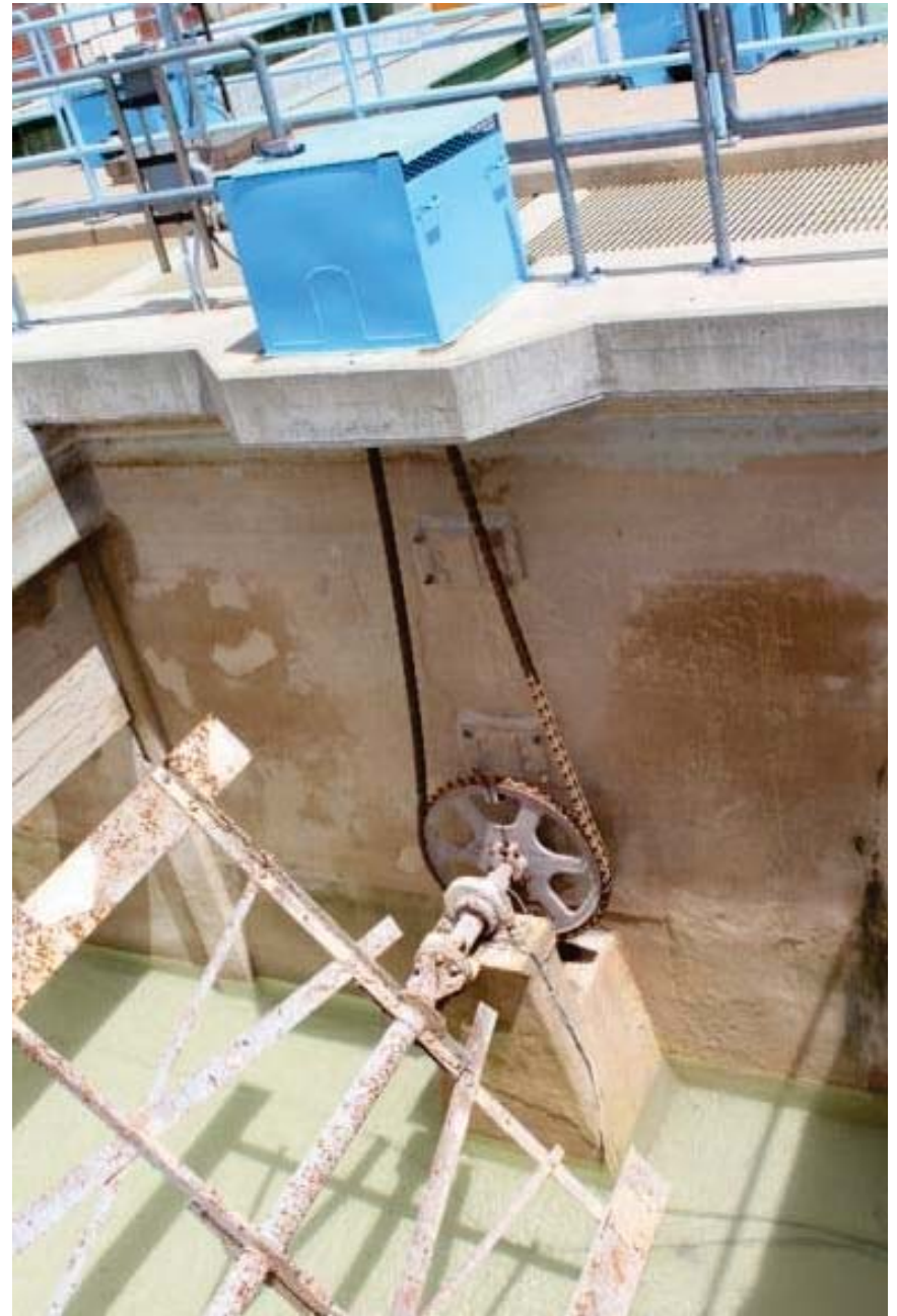
Basin No. 2 Stage 3 Flocculator Drive, Chain, and Lower Sprocket
