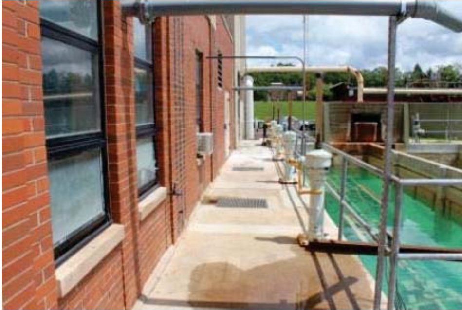
Basin No. 1 Influent Distribution Gate Actuators
