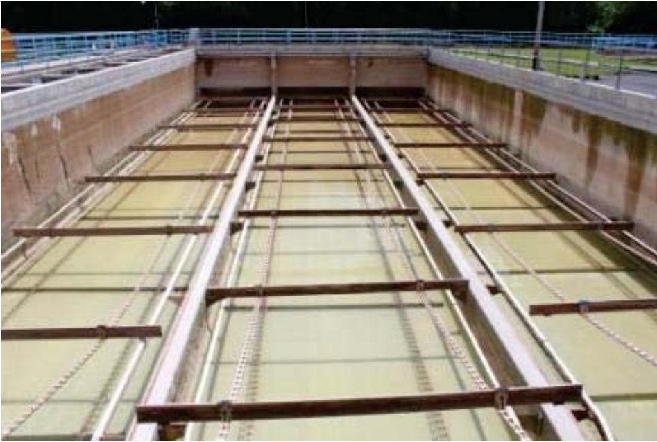
Basin No. 2 Sludge Collection Equipment
