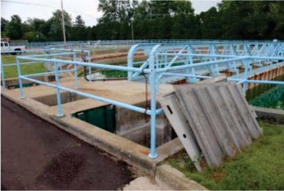
Basin No. 3 North Effluent Structure and Slide Plates
