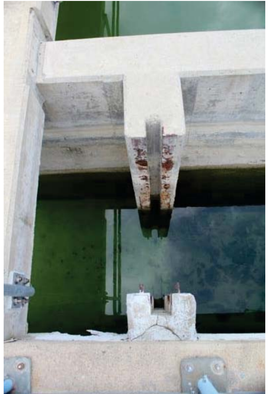
Basin Nos. 1 & 2 Effluent Stop Log Frame
