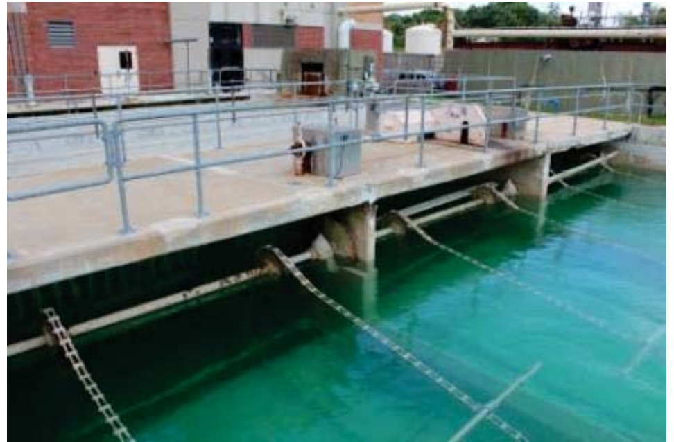
Basin No. 1 Sludge Collection Drive and Equipment
