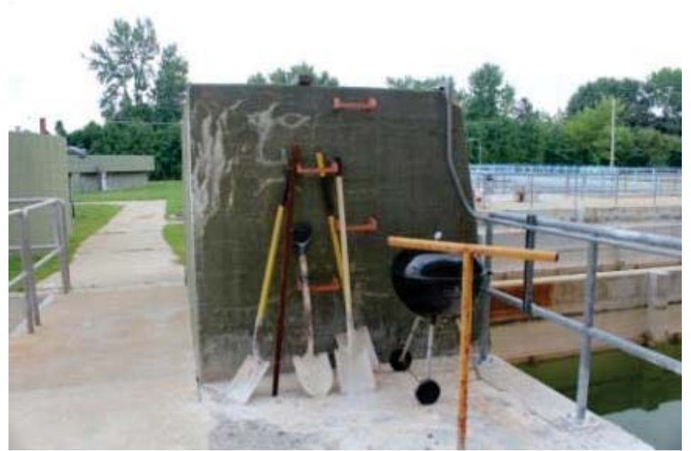
Well Water Influent Chamber/Overflow
