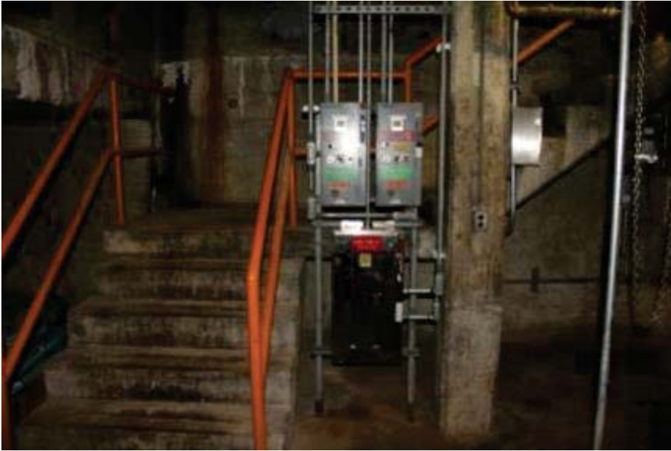
Sludge Pumps 3 & 3A and Drain Pump 2 Electrical/Control
