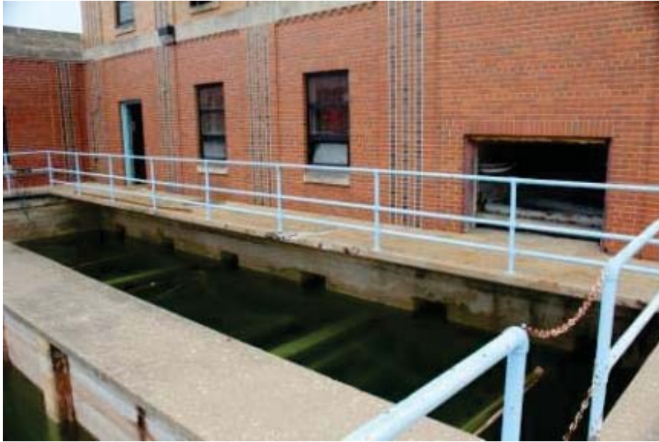
Flocculation Basin No. 3 Stage 1
