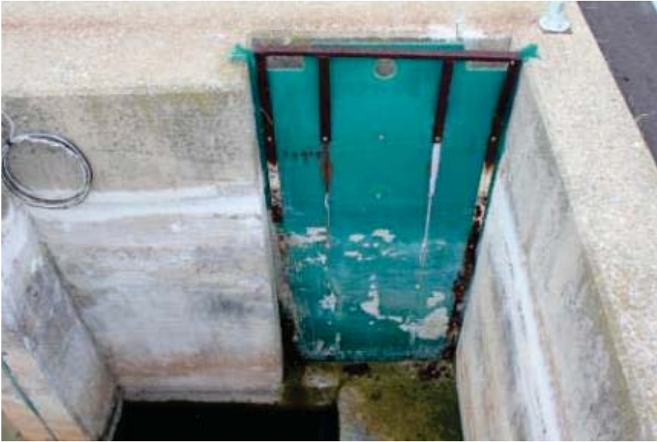
Basin No. 3 North Effluent Structure and Slide Plate
