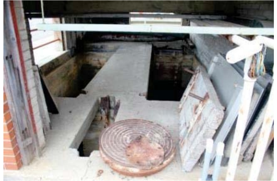
Flocculation Basin No. 3 Recarbonation Chamber Stop Log Structures
