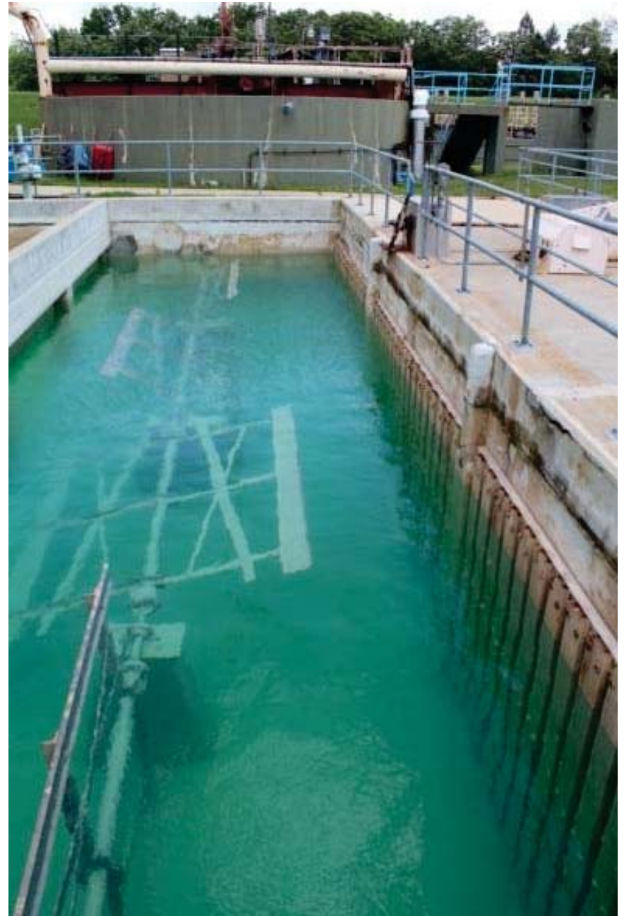
Basin No. 1 Stage 3 Flocculator and Baffle Wall
