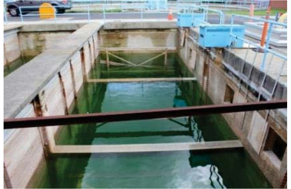
Flocculation Basin No. 3 Stage 3, Baffle Wall, and Flocculator Drives
