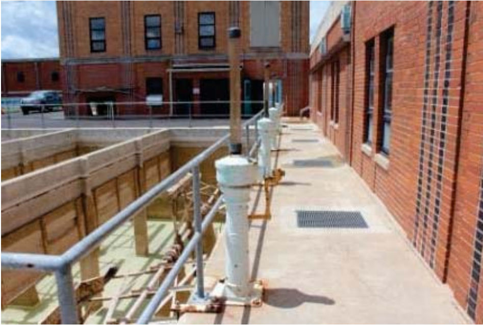
Basin No. 2 Influent Distribution Gates
