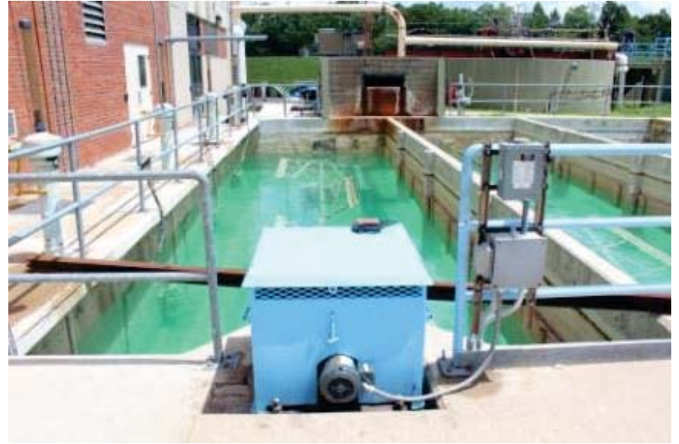
Basin No. 1 Stage 1 Flocculator Drive
