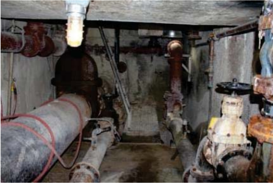
24-inch Raw Influent, 8-inch Sludge (Basin 1 & 2)
