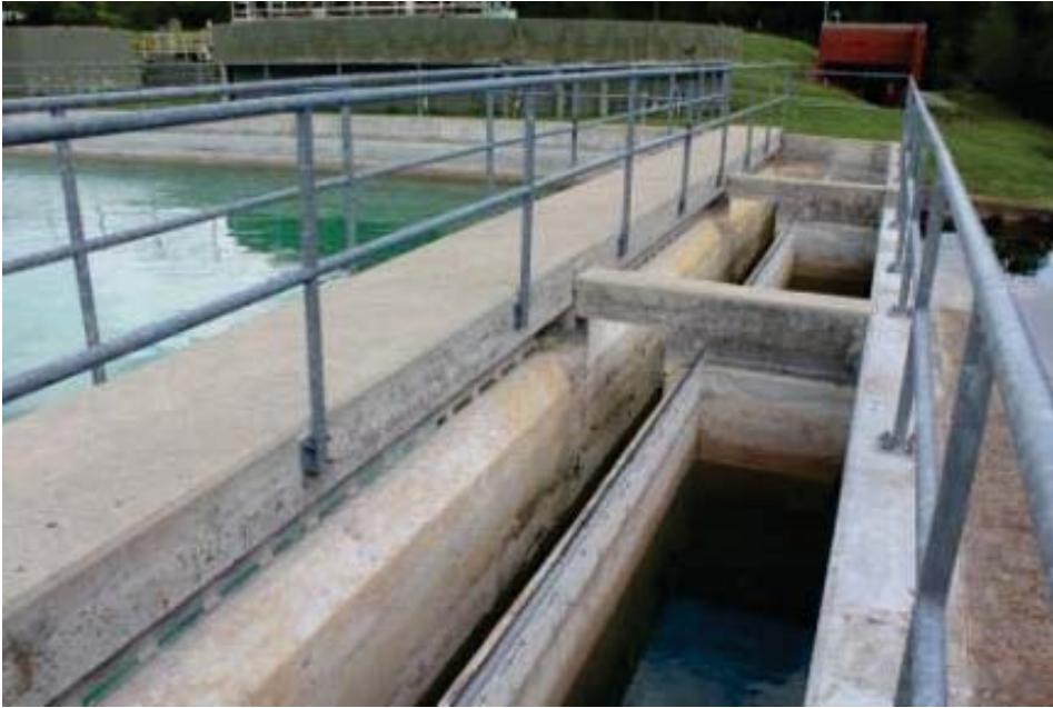
Basin No. 1 Effluent Weirs
