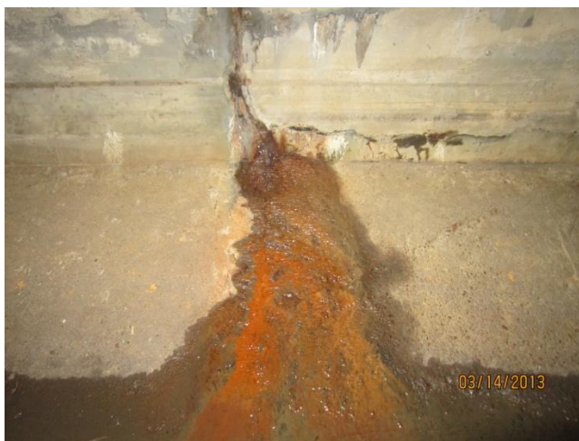
Photo 24 Station 600+20: joint leak
