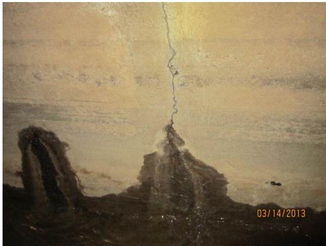
Photo 17 Station 300+5: seam leak, crack in grout
