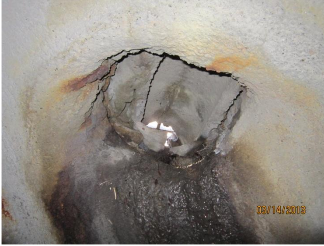
Photo 31 Station 800+20: curb inlet, poor condition
