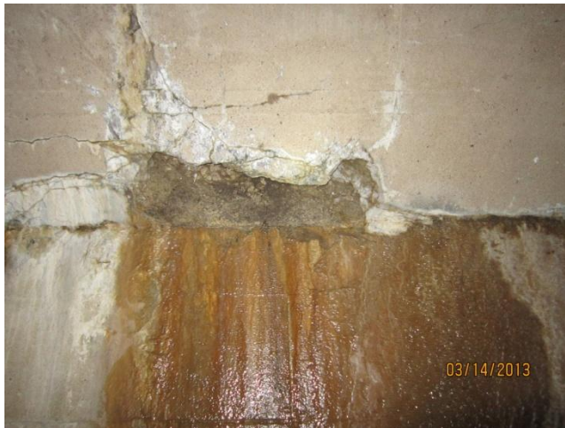
Photo 5 Station 100+65: crack in wall, seam leaking
