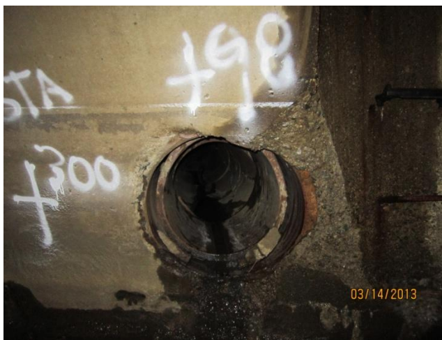
Photo 15 Station 200+98: 18" clay pipe, poor joint
