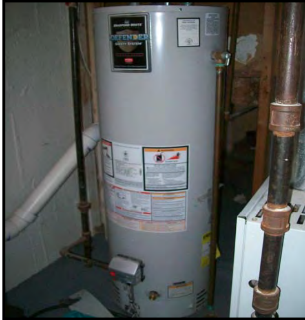
PHOTOGRAPH NO. 9: TYPICAL VIEW OF HOT WATER HEATERS IN TENANT UNITS
