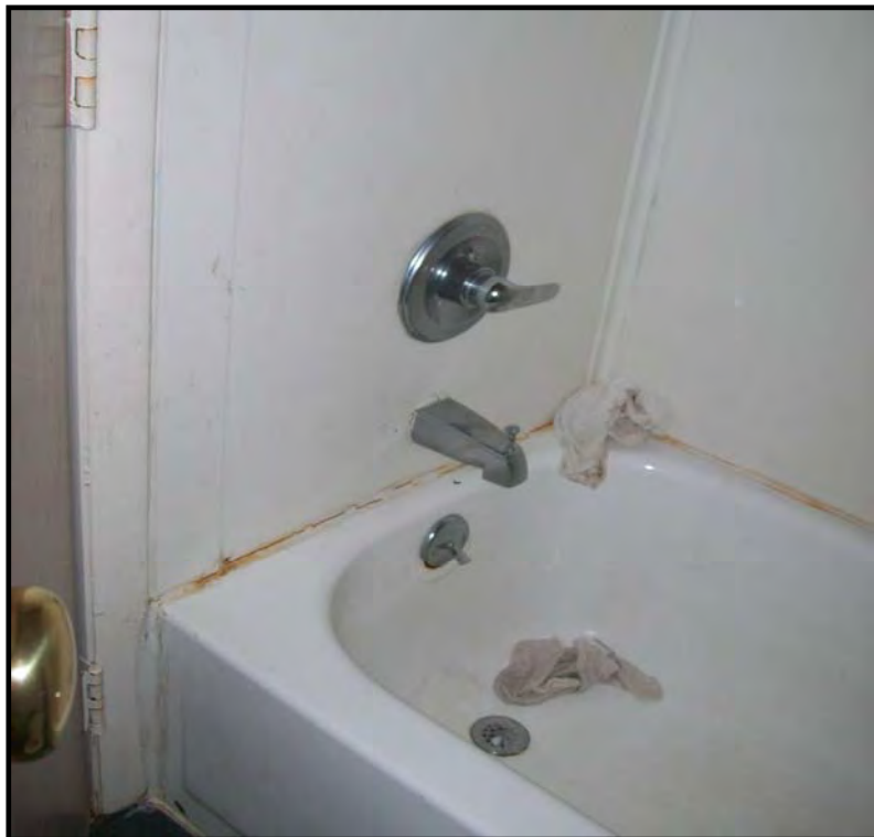
PHOTOGRAPH NO. 16: TYPICAL VIEW OF TENANT UNIT TUB AND ASSOCIATED VINYL ENCLOSURE
