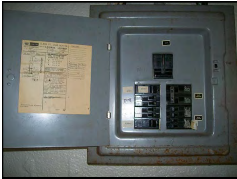
PHOTOGRAPH NO. 7: TYPICAL VIEW OF ELECTRICAL PANELS IN TENANT UNITS
