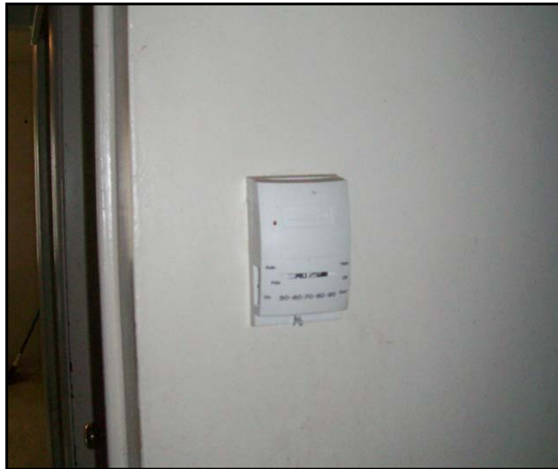
PHOTOGRAPH NO. 18: TYPICAL VIEW OF TENANT UNIT THERMOSTAT
