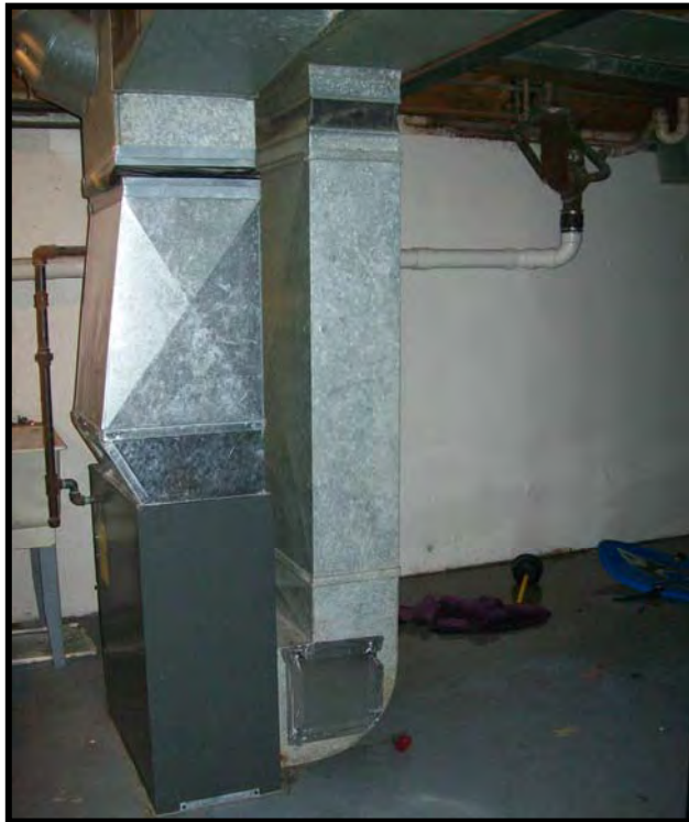
PHOTOGRAPH NO. 10: TYPICAL VIEW OF TENANT UNIT FURNACE
