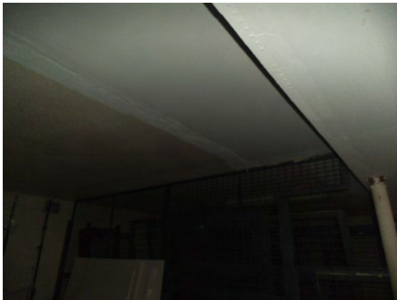
Photo 17: Mechanical storage room below units
