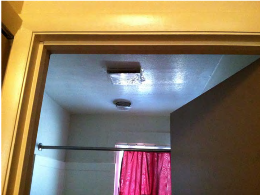
PHOTOGRAPH NO. 12: EXHAUST FAN IN BATHROOM
