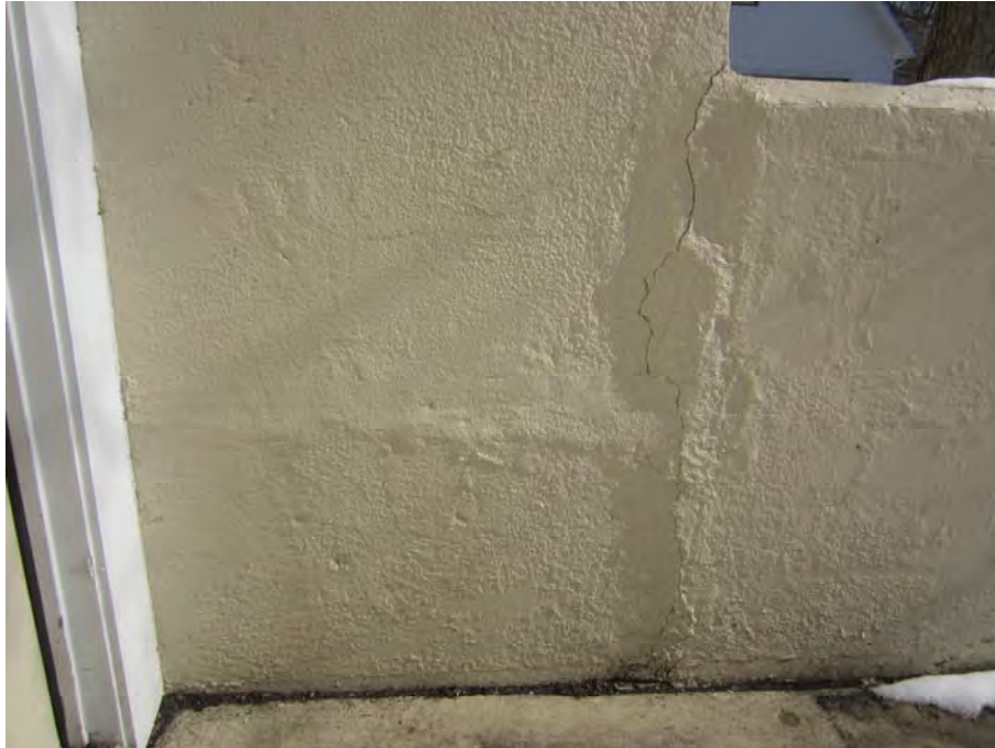
PHOTOGRAPH NO. 5: TYPICAL VIEW OF CRACKS IN RETAINING WALLS
