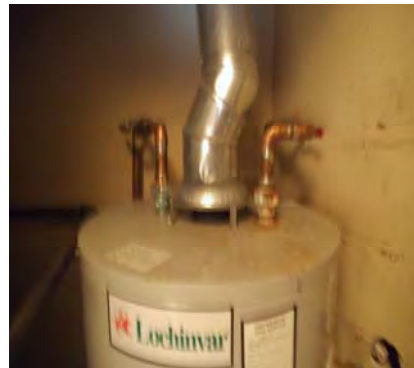
Photo 6: Typical DHW storage tank in unit
