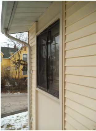
Photo 3: Older windows in need of replacement
