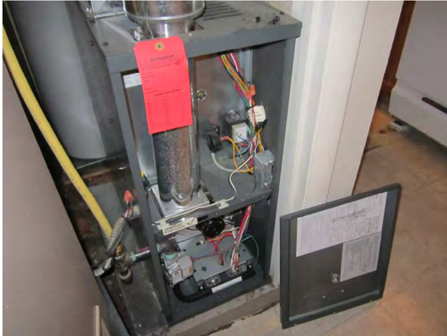
PHOTOGRAPH NO. 9: TYPICAL VIEW OF FURNACES IN TENANT UNITS (805)
