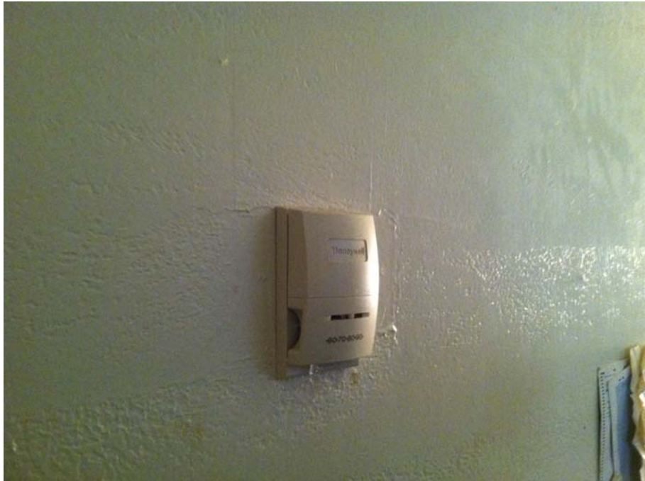
PHOTOGRAPH NO. 14: TYPICAL VIEW OF TENANT UNIT THERMOSTAT
