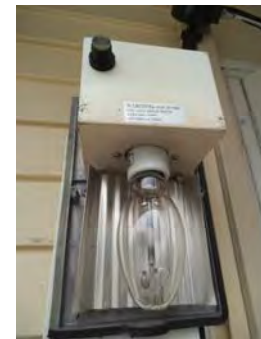
50W HPS lighting
