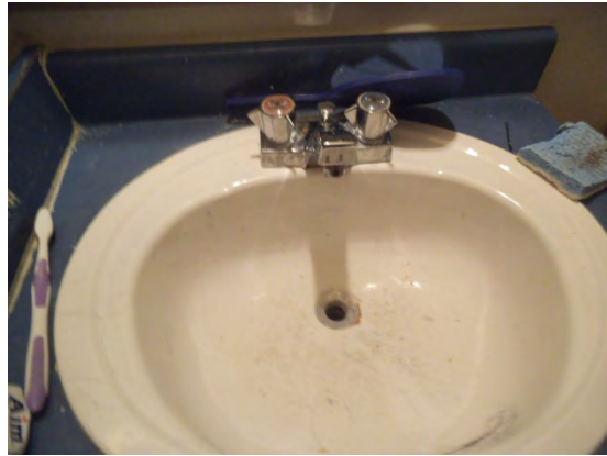
Photo 10: Faucet aerator on sink faucet bathrooms
