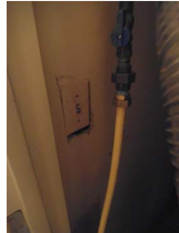
Air pathways at switch cover
