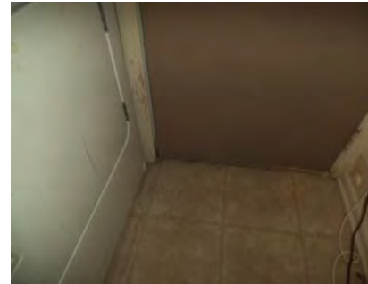
Seals worn at bottom of entry door
