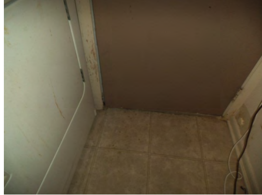
Photo 14: No weather-stripping causing leakage
