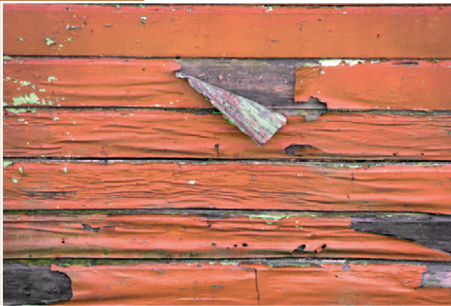
Paint in good condition does not require removal, but the peeling paint on this siding will need to be removed before repainting. Safe methods include wet scraping, wet sanding, or stripping with low heat or chemicals. Disposable tarps to collect the loose, wet paint will also be necessary. Photo source: istockphoto.com
