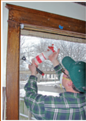
Wet scraping of some deteriorating varnish. Some varnish on old wood windows contains lead, so lead-safe practices should be used when working on these surfaces. Photo courtesy of Sharon Ferraro.
