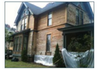
The siding on this home in Kalamazoo is being stripped. The disposable plastic sheeting catches the wet deteriorated paint. Photo courtesy of Sharon Ferraro.
