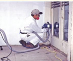
Top: Plastic sheeting in this doorway keeps dust in the work area while allowing workers access. Photo courtesy of Sharon Ferraro.
