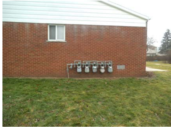
Photo 2: Utility meters on side of complex
