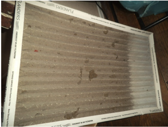
Photo 13: Old furnace filter
