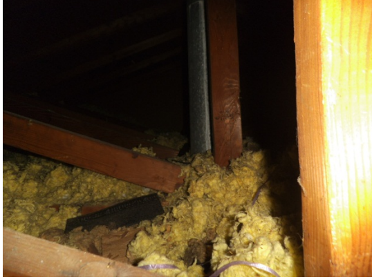
Photo 13: Fiberglass blown insulation in attic
