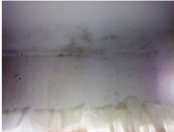
Photo #25: Unit 3681 Water damage in bathroom
