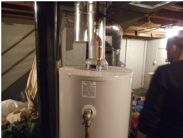
Photo 11: Residential DHW storage tank in basement
