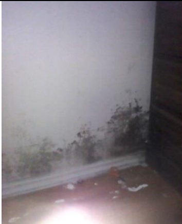
Photo #27: Unit 3681 Moisture damage in bedroom 2
