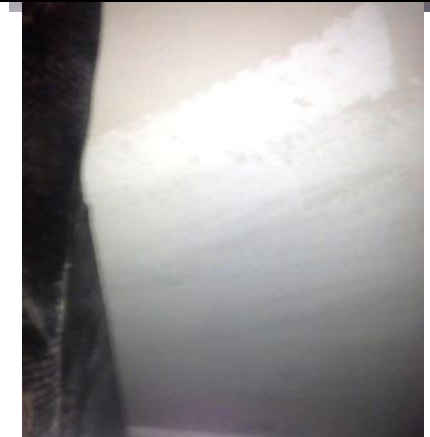
Photo #28: Unit 3681 Moisture damage in bedroom 3 covered with paint
