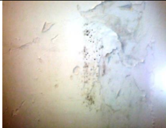
Photo #24: Unit 3681 water damage in basement
