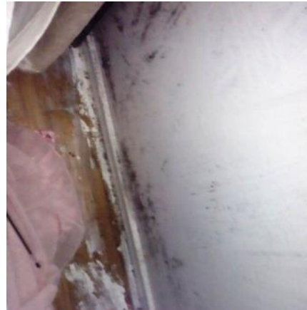
Photo #26: Unit 3681 Moisture damage in bedroom 1
