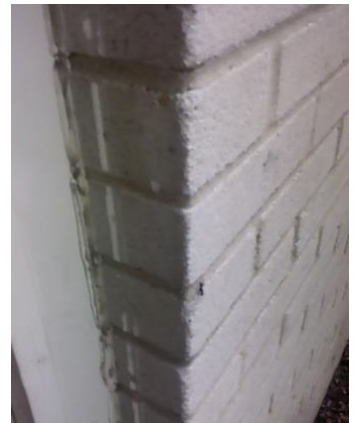
Photo #29: Carpenter ant crawling up doorway of unit 3681 with all the moisture damage.
