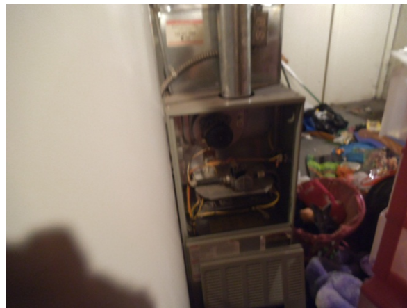
Photo 12: Interior of furnace in basement
