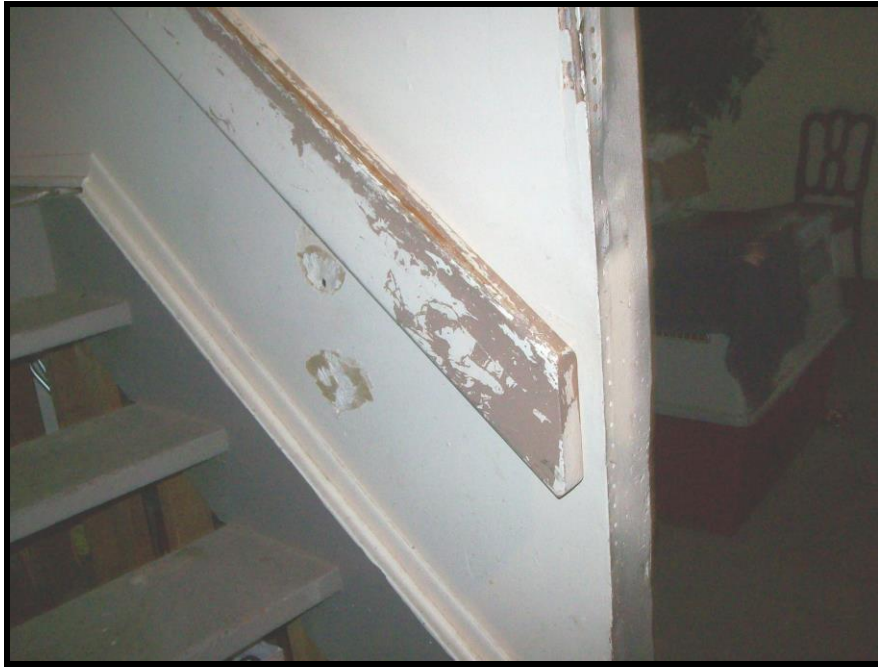
PHOTOGRAPH NO. 19: VIEW OF DAMAGED DRYWALL AND PAINT IN TENANT UNIT
