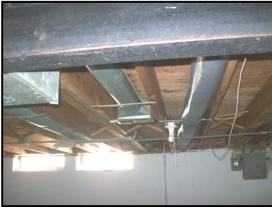
PHOTOGRAPH NO. 13: TYPICAL VIEW OF DUCTWORK AND JOIST BRACING IN TENANT UNIT BASEMENT
