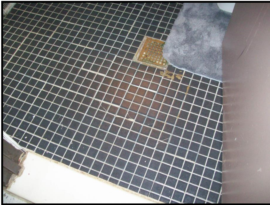
PHOTOGRAPH NO. 15: TYPICAL VIEW OF FLOORING IN TENANT UNIT BATHROOMS
