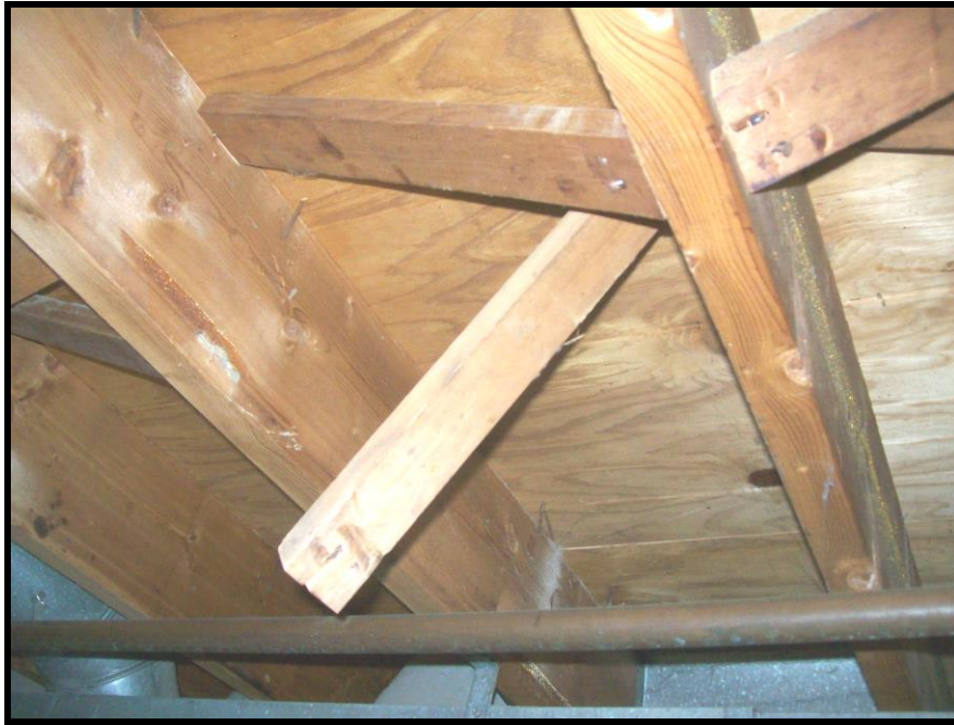
PHOTOGRAPH NO. 21: VIEW OF DAMAGED JOIST BRACING IN TENANT UNIT
