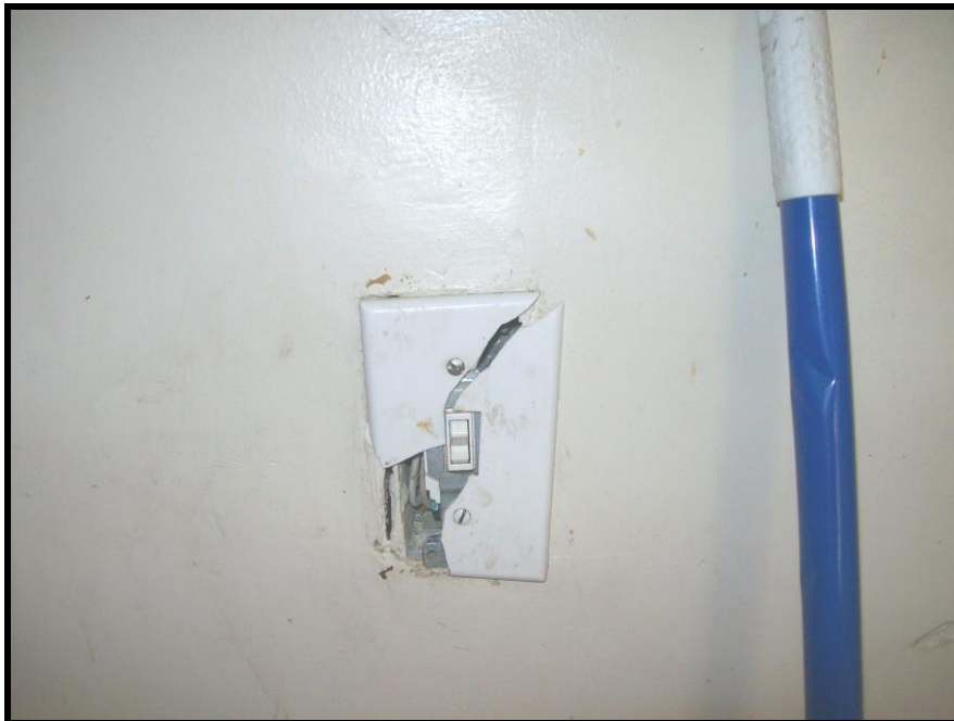
PHOTOGRAPH NO. 22: VIEW OF DAMAGED ELECTRICAL SWITCH COVER IN TENANT UNIT
