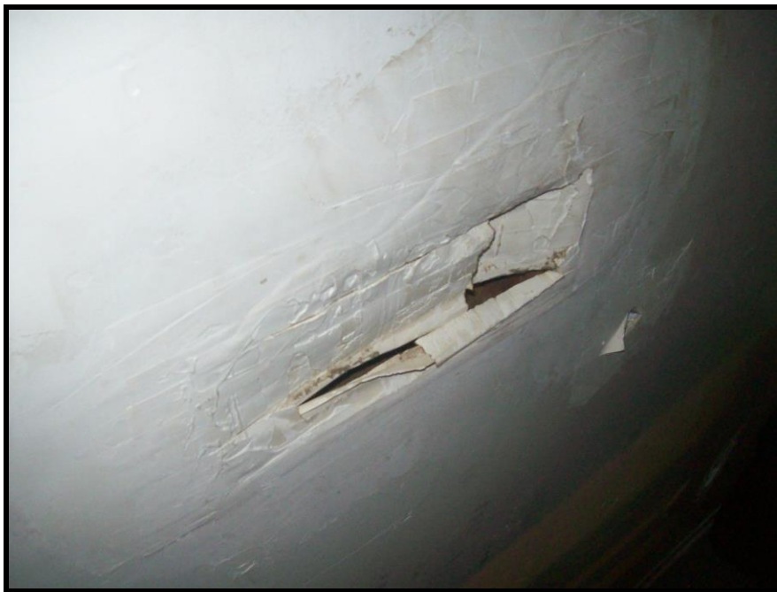
PHOTOGRAPH NO. 18: DAMAGED DRYWALL IN TENANT UNIT
