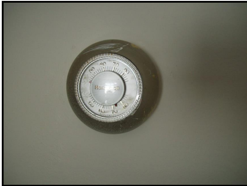
PHOTOGRAPH NO. 20: TYPICAL VIEW OF TENANT UNIT THERMOSTAT
