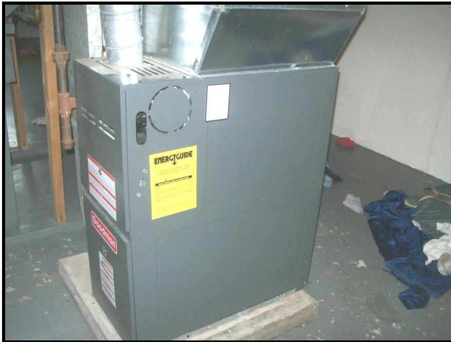
PHOTOGRAPH NO. 12: TYPICAL VIEW OF TENANT UNIT FURNACE
