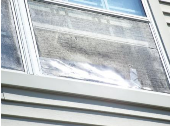
Photo #19: Damaged window screens (there is tape over holes currently)
