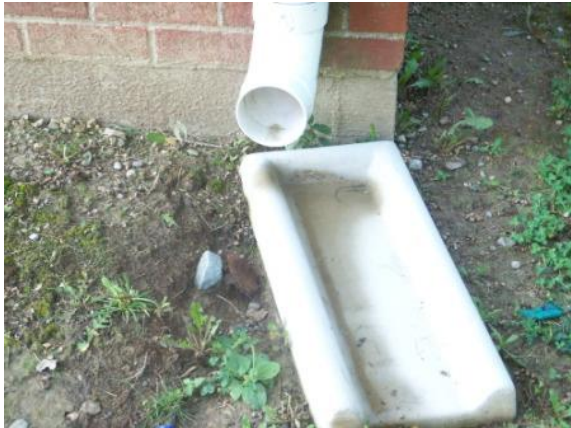
Photo #25: Offset downspout, water will pool at foundation.
