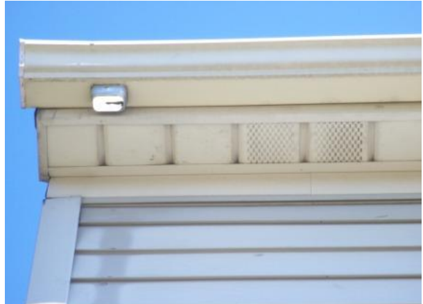
Photo #190: Missing downspout
