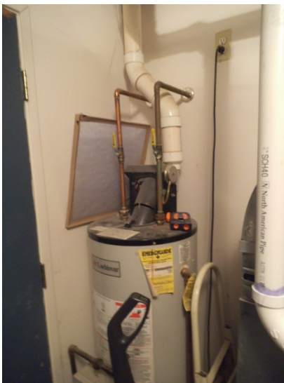
Photo 17: DHW tank in mechanical room
