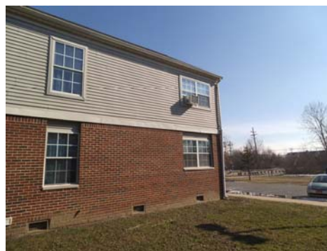
Second floor AC unit
