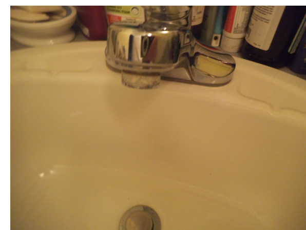
Photo 12: Bathroom faucet with aerator
