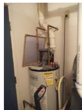
Uninsulated HW pipe/tank
