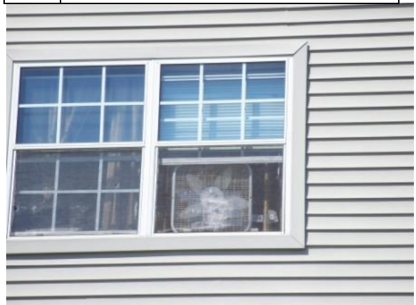
Photo #18: Damaged window screens
