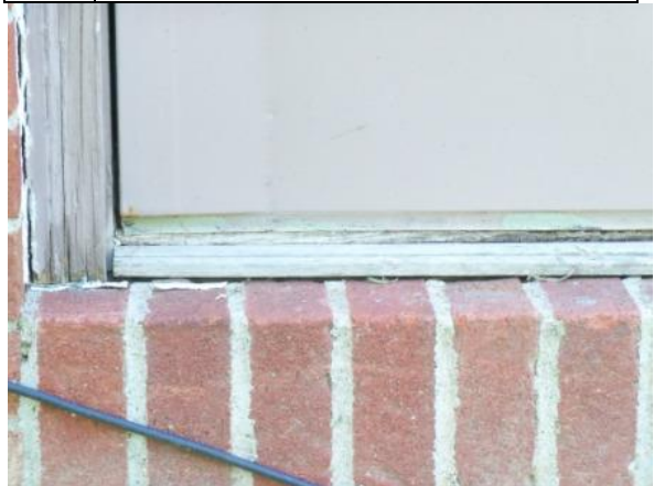
Photo #22: Gap around door, potential entry point
