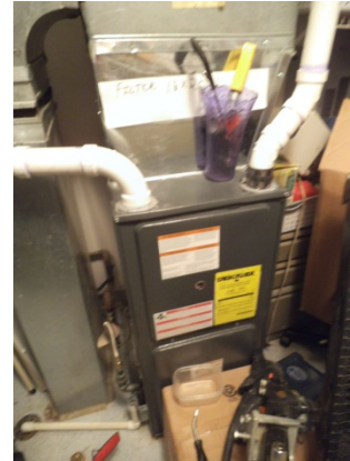
Photo 16: High Efficiency Furnace in mechanical rm.
