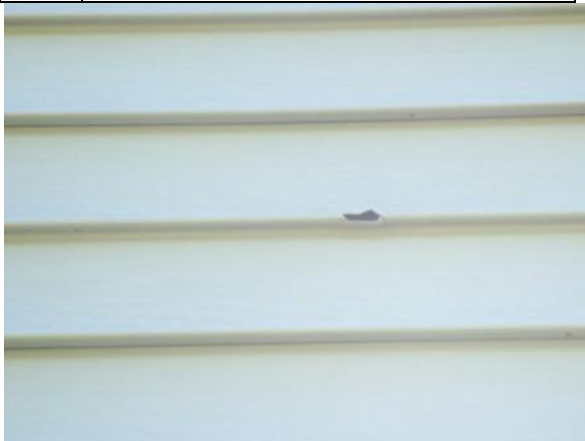
Photo #21: Holes in siding, potential entry point
