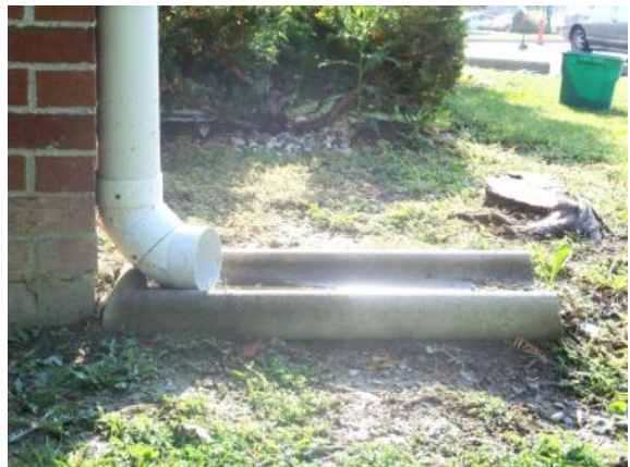
Photo #24: Downspout not sloping away from building. Water will pool at foundation.
