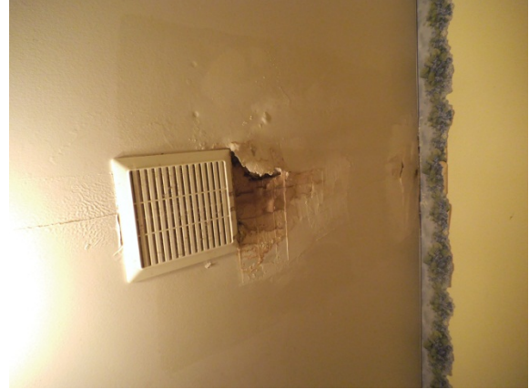
Photo 14: Bathroom exhaust fan (water damage)
