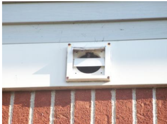
Photo #23: Damaged dryer vent, Potential entry point
