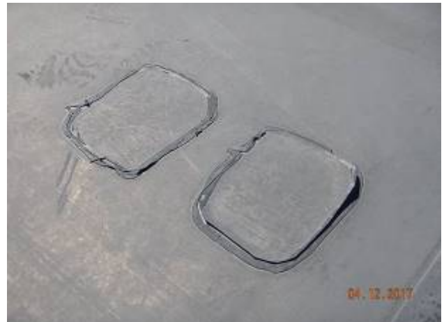
Superior Hydroelectric Pumping Station Deficient adhesion of roof membrane patches.
