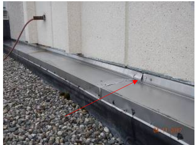
Control Rooms – CR-2 Overview of metal closure piece. Note lifting of metal, needs to be re-secured/sealed.
