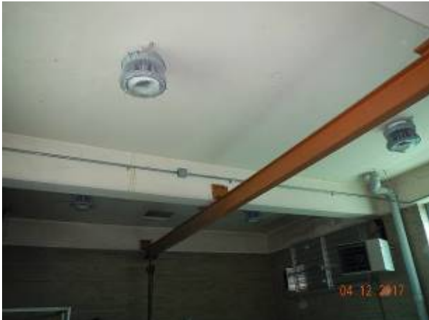
Industrial Pumping Station
