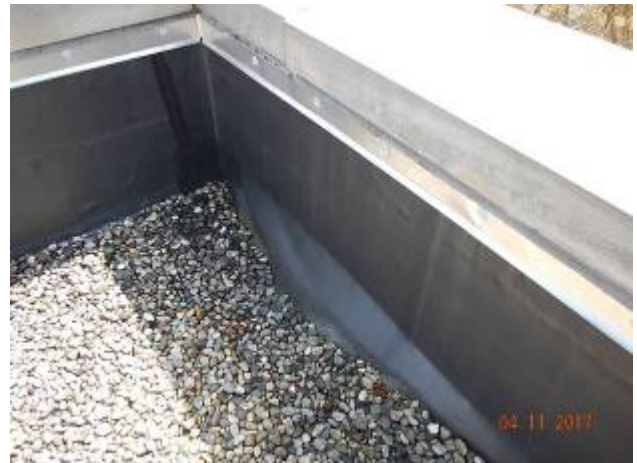
Ozone Building – OZ-1 Base flashing delamination due to deficient adhesion.
