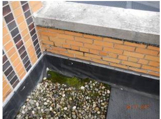
Control Rooms – CR-1 Vegetative growth on roof surface. Note masonry wall mortar deterioration.
