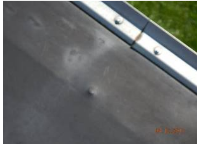
North Campus Pumping Station Fastener backout at perimeter edge base flashing and will create holes in the roof system.
