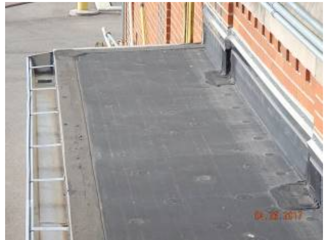
Carbon House – CH-2 Minor surface erosion throughout.
