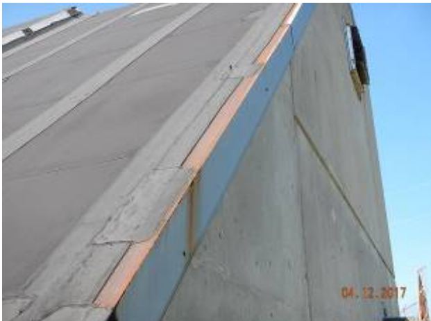
Superior Hydroelectric Pumping Station Rust at perimeter edge metal.
