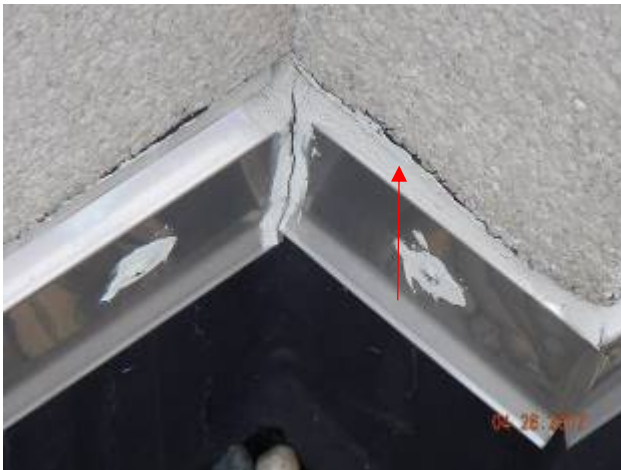
Filter Press – FP-1 Deteriorated sealant at top of counterflashing.
