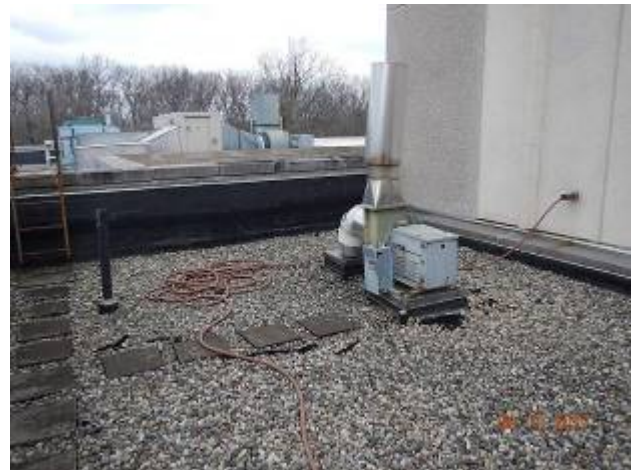
Control Rooms – CR-2
