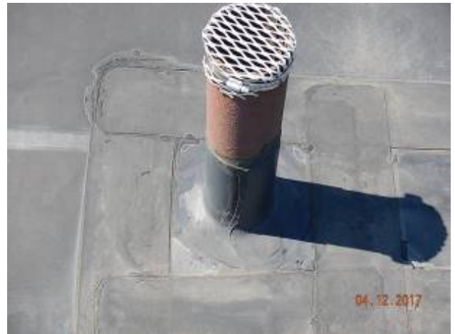
North Campus Pumping Station Rust corrosion at pipe.
