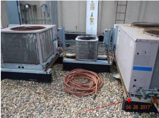
Filter Press – FP-1 Rust at roof top unit curbs.
