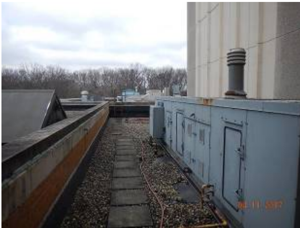
Control Rooms – CR-2
