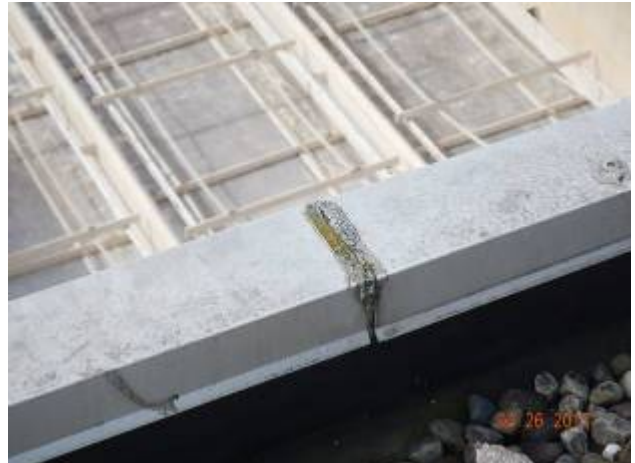
Calciner Building – CA-1 Deteriorated sealant at metal coping seam.
