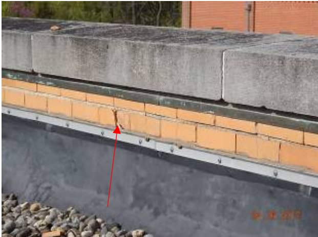
Carbon House – CH-1 Flaking of brick masonry indicating signs of moisture infiltration.
