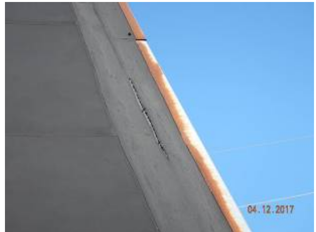
Superior Hydroelectric Pumping Station Splitting at base flashing strip-in and rust along perimeter edge metal.
