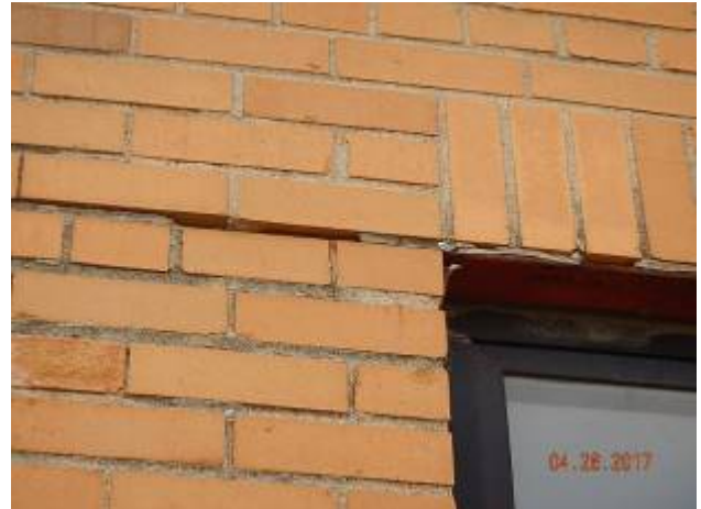
Carbon House – CH-1 Deterioration of mortar at brick masonry wall.
