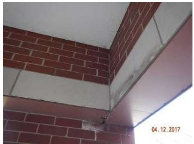
Admin Building – AD-2 Signs of leakage at lintel below roof system. Additional evaluation of masonry recommended.
