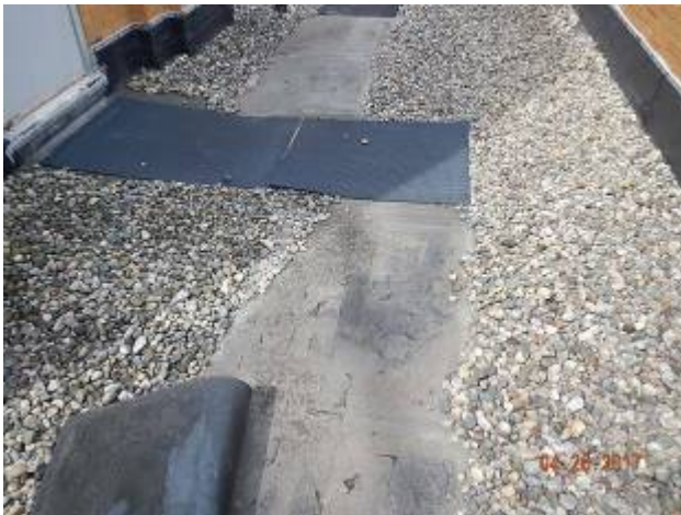
Penthouse – P-1 Missing/loose walkpads preventing foot traffic protection.
