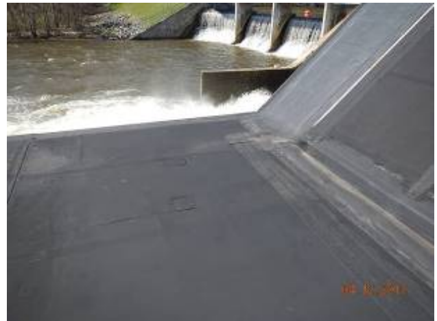
Superior Hydroelectric Pumping Station
