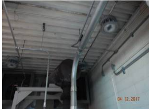
Industrial Pumping Station
