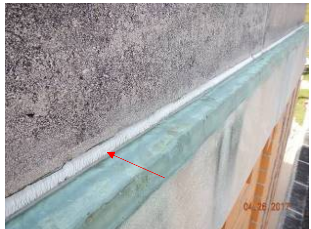
Carbon House – CH-1 Deteriorated sealant at base of stone coping.
