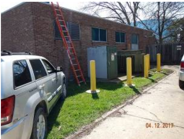
Industrial Pumping Station
