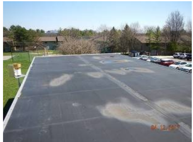
North Campus Pumping Station Overview of the roof area. Note spots of ponding water.
