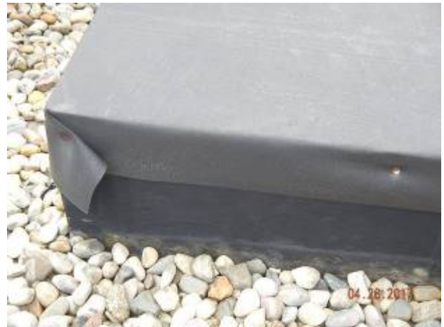
Filter Press – FP-1 Temporary flashing membrane cover over obsolete curb. Recommend installing a permanent metal cover or removing and decking over.
