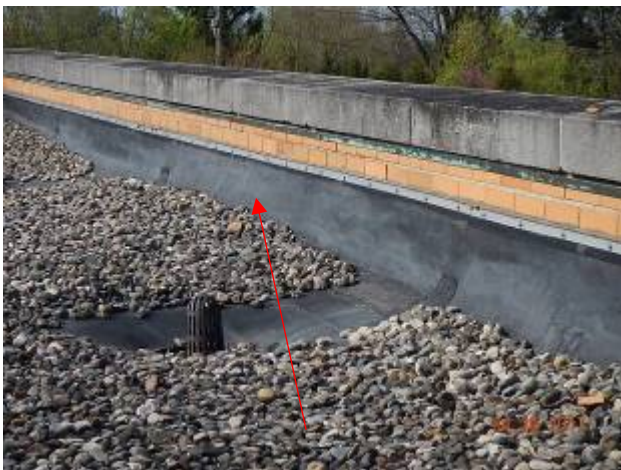
Carbon House – CH-1 Base flashing pulling from wall showing old age of roofing system.
