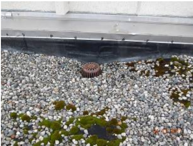
Control Rooms – CR-2 Vegetation growth on roof surface. Remove vegetation to prevent any potential root penetration in roof surface.
