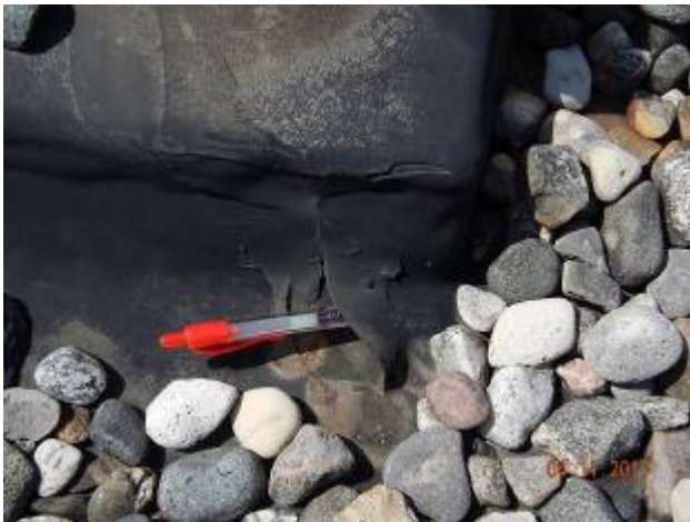
Ozone Building – OZ-1 Open base flashing seam allowing potential water infiltration.
