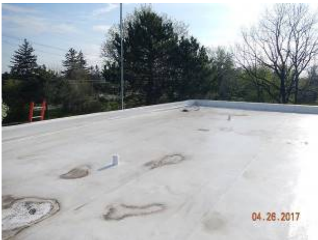
Liberty Pumping Station Overview of the roof area. Note spots of ponding water throughout.
