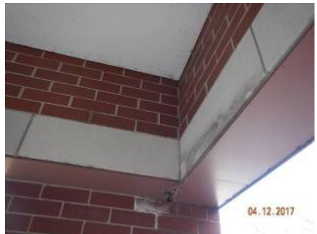
Admin Building – AD-2 Signs of leakage at lintel below roof system. Additional evaluation of masonry recommended.
