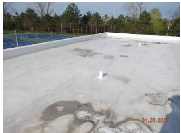
Liberty Pumping Station Overview of the roof area. Note spots of ponding water throughout.
