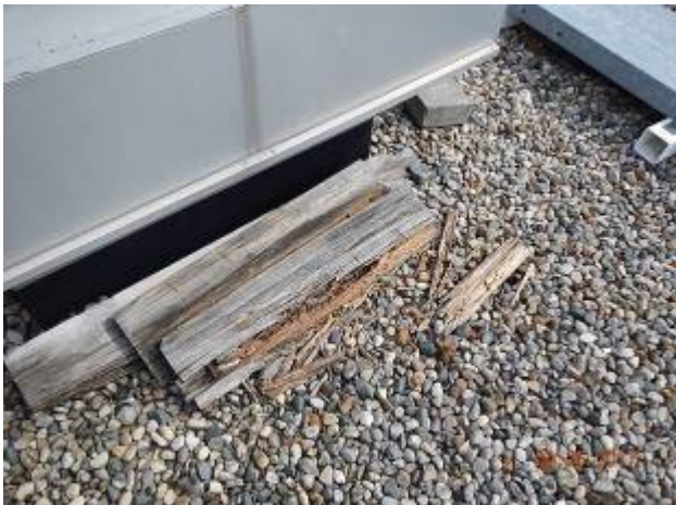
Calciner Building – CA-1 Debris on roofing surface.
