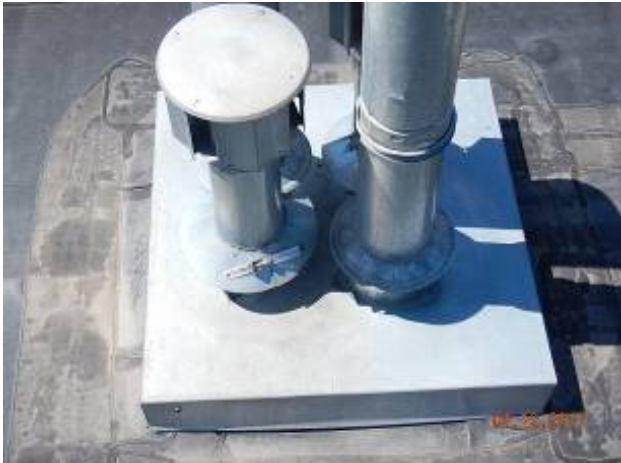
North Campus Pumping Station Low flashing height at pipe projection curb.
