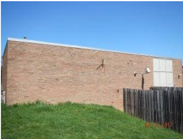
North Campus Pumping Station Overview of the north campus pumping station.
