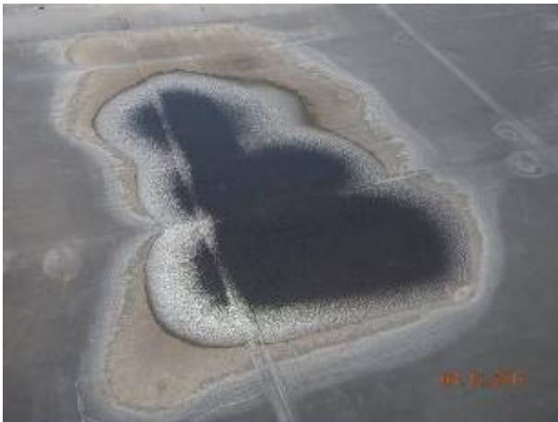
North Campus Pumping Station Ponding water on roof surface.
