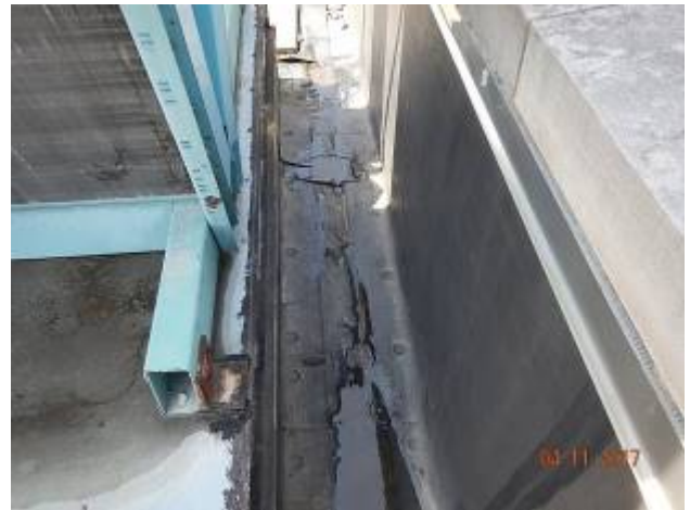
Admin Building – AD-1 Ponding water noted due to lack of slope at wall.
