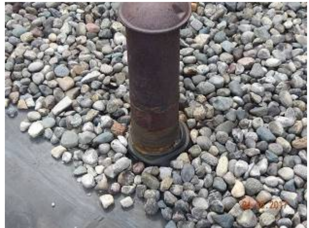
Penthouse – P-1 Deteriorated sealant at pipe boot and clamping ring. Note rusted pipe projection.
