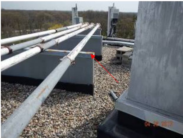
Calciner Building – CA-1 Rust and paint failure at conduit pipe supports.
