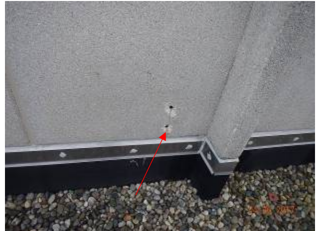
Filter Press – FP-1 Exposed/rusted fasteners at wall panel.
