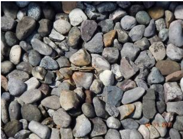
Admin Building – AD-1 Shaling of ballast creating sharp objects that can penetrate the roof system.
