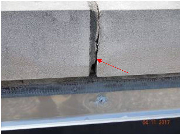
Ozone Building – OZ-1 Deterioration of mortar at coping joint.
