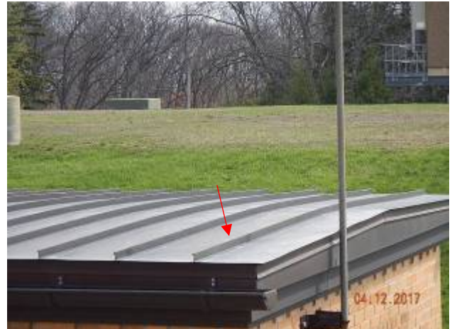
Ammonia Building – A-1 Minor spots of coating deterioration.
