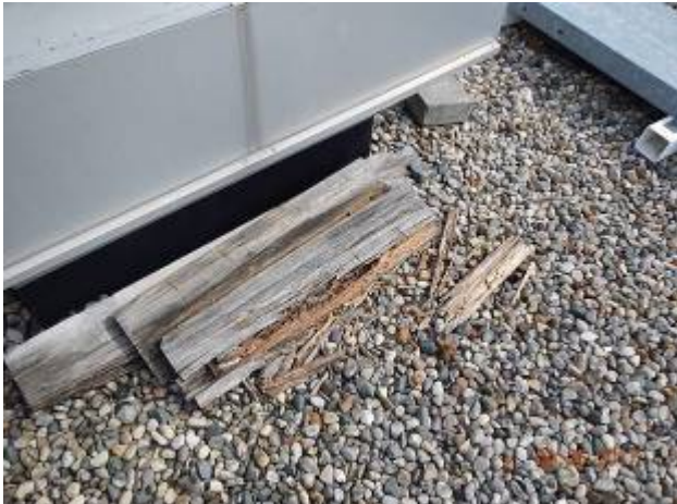
Calciner Building – CA-1 Debris on roofing surface.
