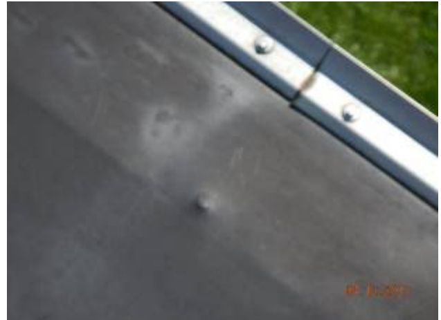
North Campus Pumping Station Fastener backout at perimeter edge base flashing and will create holes in the roof system.
