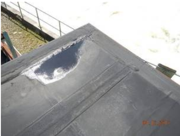
Superior Hydroelectric Pumping Station Ponding water at perimeter edge.
