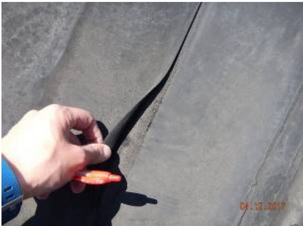
Superior Hydroelectric Pumping Station Deficient adhesion of membrane seams.
