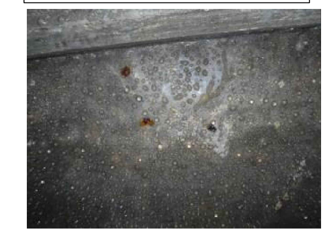
D COAT REBAR AND PATCH CONCRETE SPALLS INSIDE WET INTERIOR (SEE NOTE 3)
