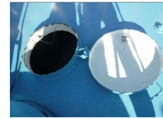
WET INTERIOR ROOF HATCH
