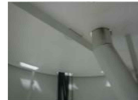
OVERFLOW PIPE AND CONDENSATE DRAIN
