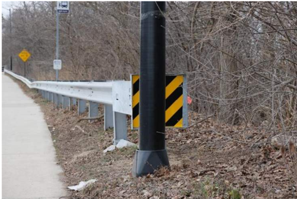
Figure 89: A light pole is located in front of the attenuator at Fuller Road and Maiden Lane intersection.
