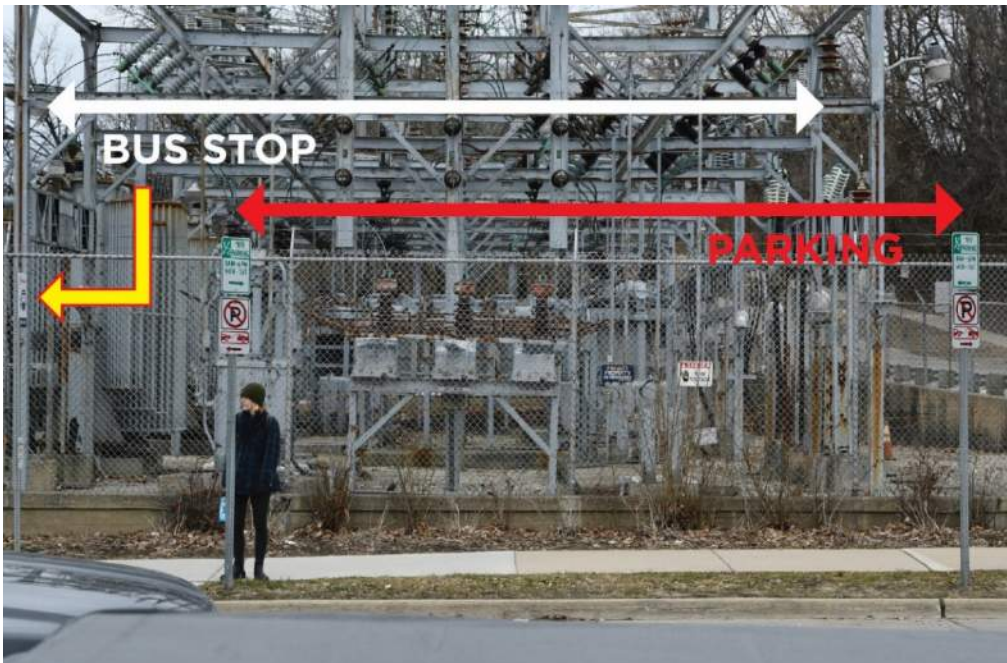
Figure 123: In front of the electrical substation on Broadway Street at Swift Street a 30-minute parking sign shares the same places as an AAATA bus stop. If a vehicle is parked in the spot, bus riders will be forced to enter the street in order to board. There is no ramp down from the sidewalk to the street level for a person in a wheelchair to travel down to the street.
