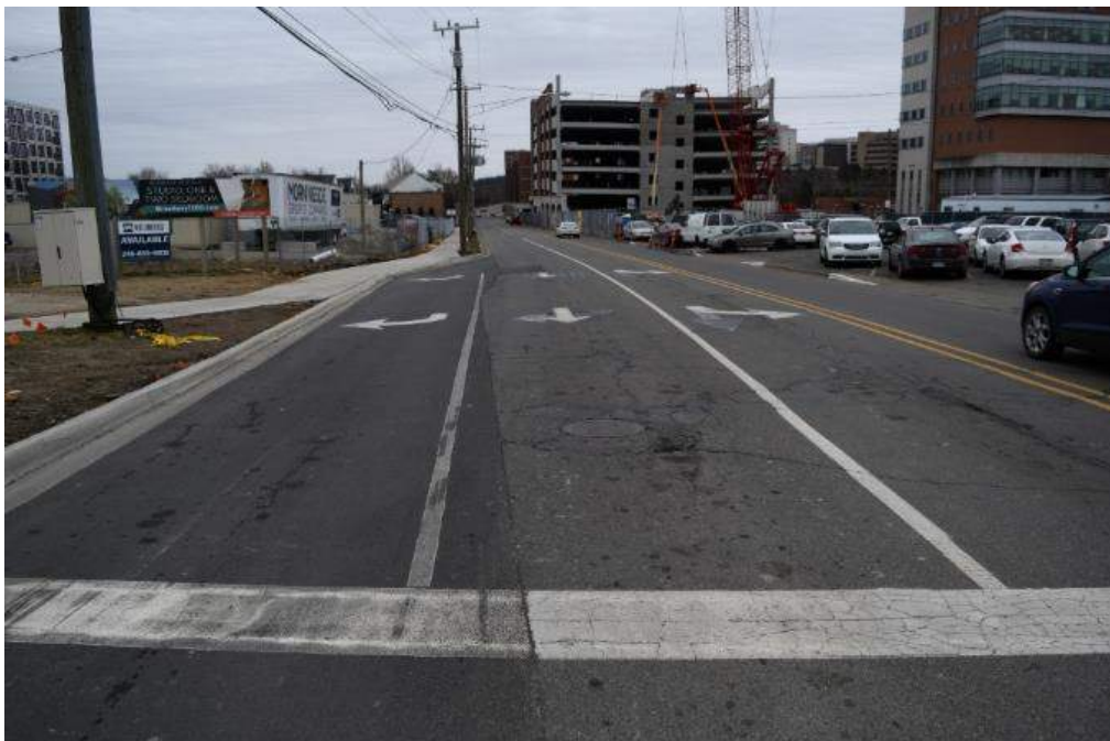
Figure 78: Old pavement markings have not been fully removed in areas where changes have been made, which sends mixed messages to road users.
