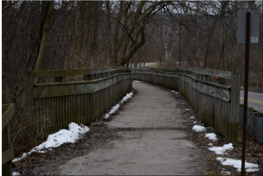
Figure 51: Shared use path boardwalk along Barton Drive, between Longshore Drive and M-14, does not meet the design standards for width. Clear width of path between railings is less than 10'. Should be ~14' per AASHTO guidelines.
