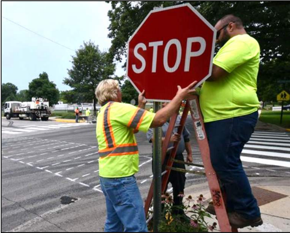
Figure 76: Inventory all signs in the study area and upgrade signs as needed.
