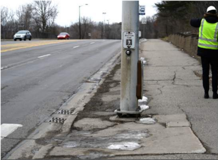
Figure 21: Crossing Ramp Lacking Detectable Warning
