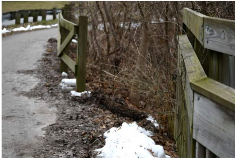
Figure 28: Gap in Fence, Coinciding with Pedestrian Desire Line to go from Barton Dr to Pathways Along Huron River
