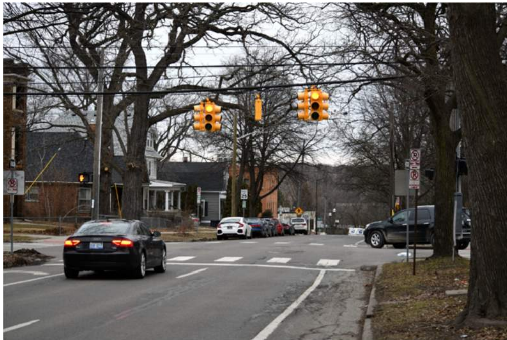
Figure 83: Outdated diagonal span-wire mounted traffic signals should be considered for modernization.
