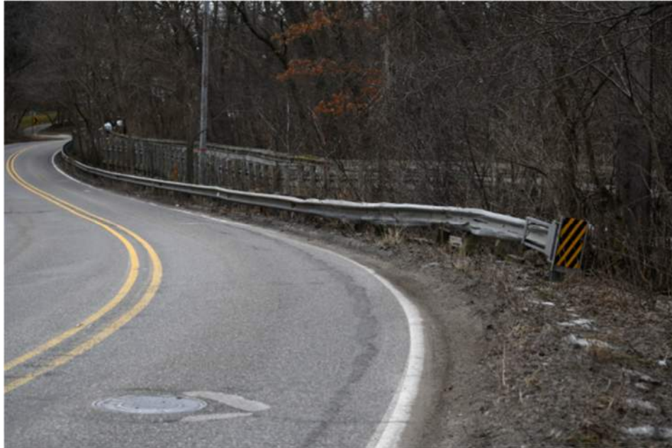
Figure 88: Guardrail is damaged at Barton Drive and M-14.
