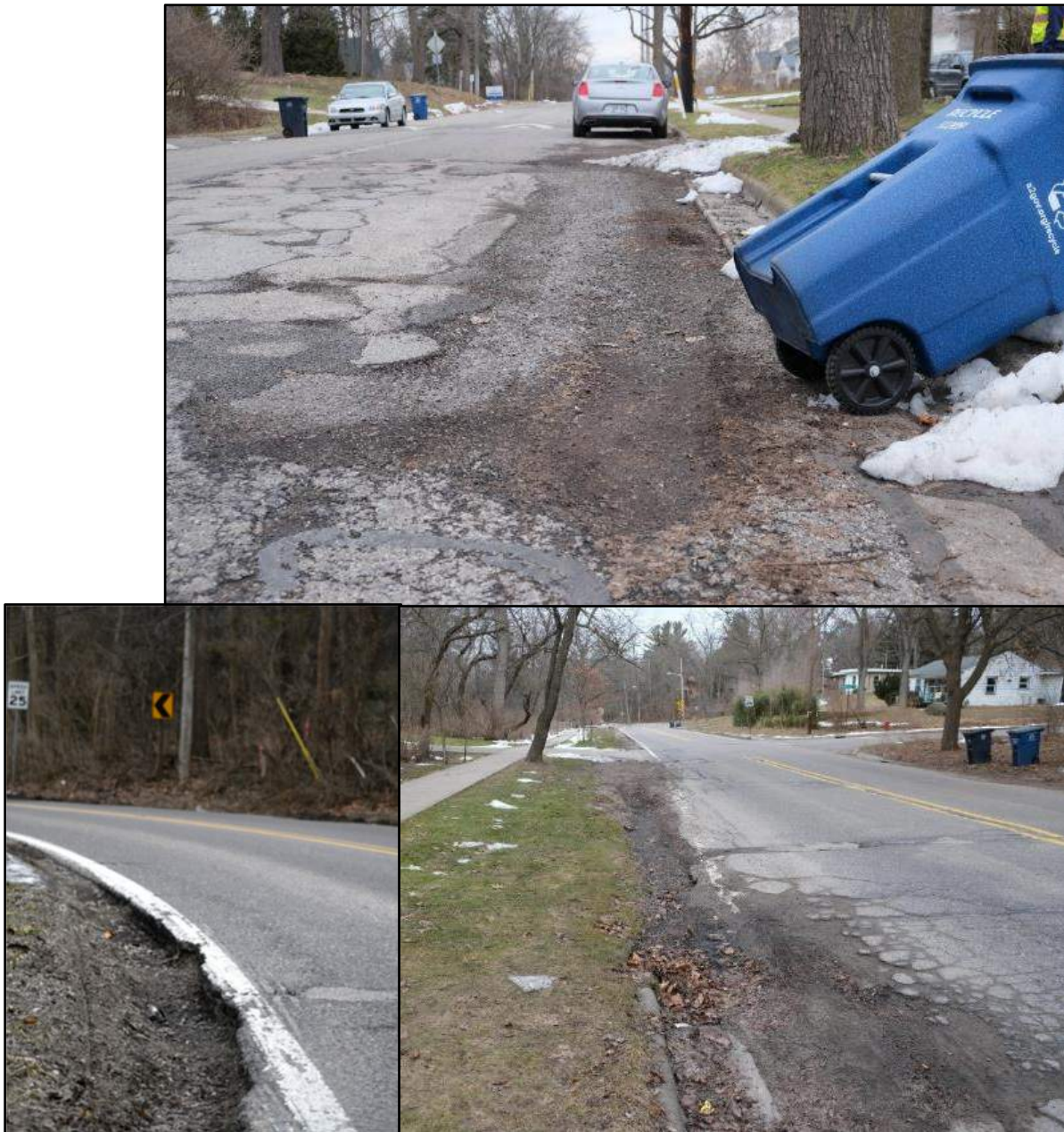
Figure 65: Poor pavement conditions, including severe edge rutting, exist on several roads within the project study area, including Broadway Street, Barton Drive, and Traver Road.
