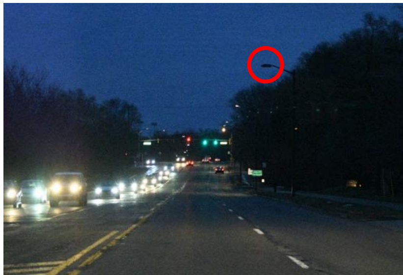
Figure 125: There is a light burned out on Plymouth Road, between Broadway Street and Barton Drive
