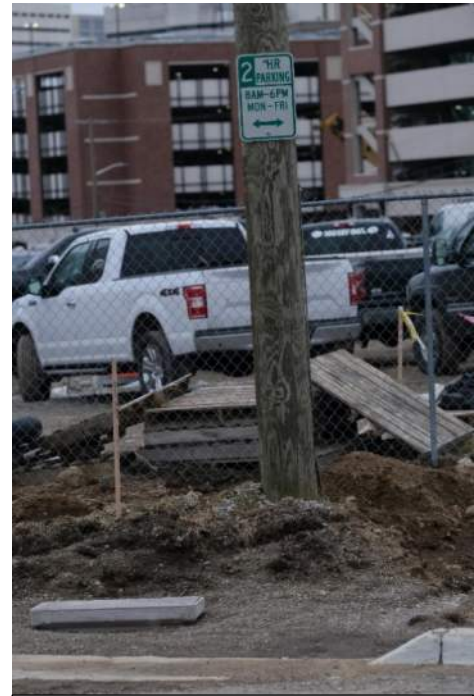
Figure 121: Other construction site issues including missing sidewalks, holes in the concrete, and exposed electrical boxes.
