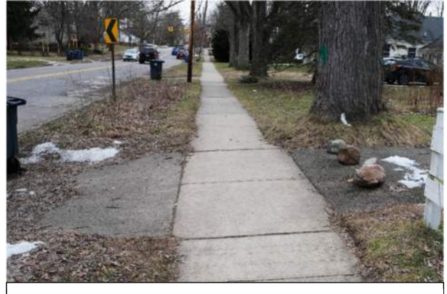
Figure 127: It is our understanding that local ordinance calls for driveway not in use to be closed. If correct, this driveway on Barton Drive is a candidate for removal.
