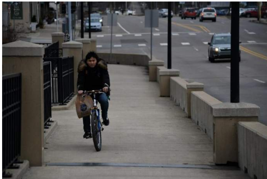
Figure 52: Broadway Street bridge has poor visibility around the curve at Division Street and concrete pillars holding light poles extend too far into the travel way. Concrete fillers should be placed to eliminate the protrusions of the bridge and lighting posts, presenting a smooth barrier face to cyclists.
