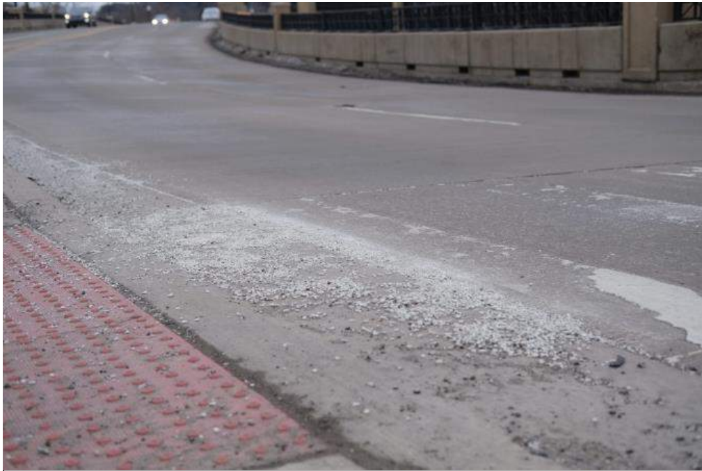
Figure 79: Multiple crosswalks throughout the Study Area have degraded markings, making it hard to distinguish where the crosswalk is.
