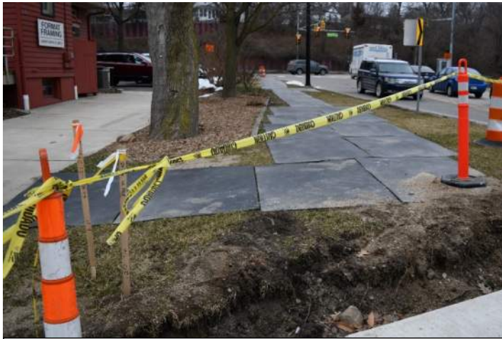
Figure 120: On Broadway, in front of the Format Framing building, a temporary sidewalk was constructed using thick rubber mats. These were not placed close enough together to eliminate gaps and the mat itself was not sturdy enough to be stable for someone in a wheelchair or walker. Caution tape was used to prevent pedestrian from falling off the end of the mat pathway at the drop off.
