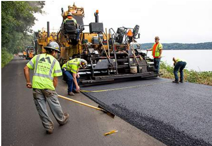
Figure 66: Rehabilitate or reconstruct pavement in areas with damaged roadway surfaces.
