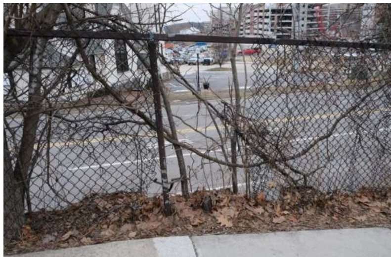
Figure 29: Gap in Fence Along Traver St Near Moore St
