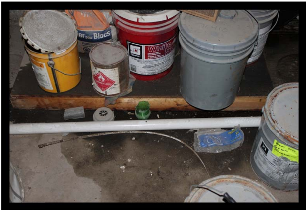
Stained concrete near miscellaneous buckets in the South Garage
