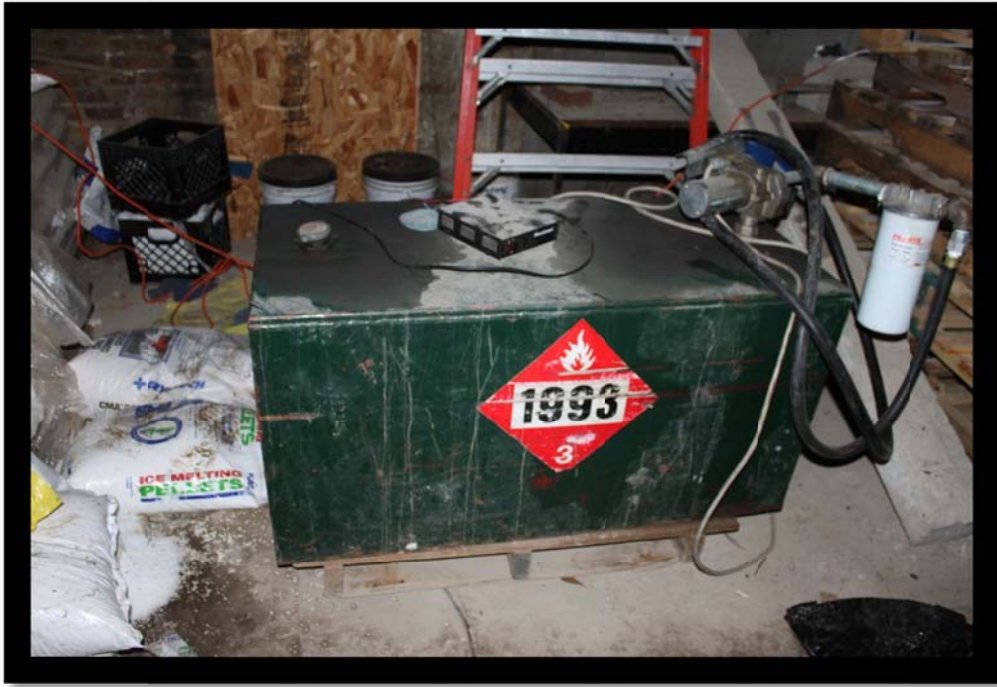
Portable diesel tank located in the South Garage
