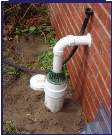
Atrium Air Gap
