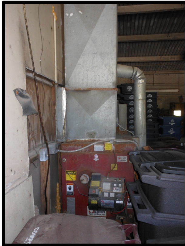
Oil burning furnace on the north wall of the southern portion of the maintenance garage
