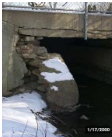
Close up of Old Stone School Road bridge damage
