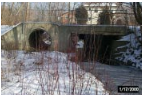
Old Stone School Road bridge in need of repair
