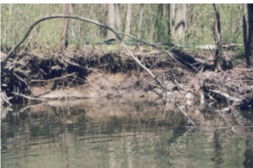
Severe bank erosion at Chalmers Road
