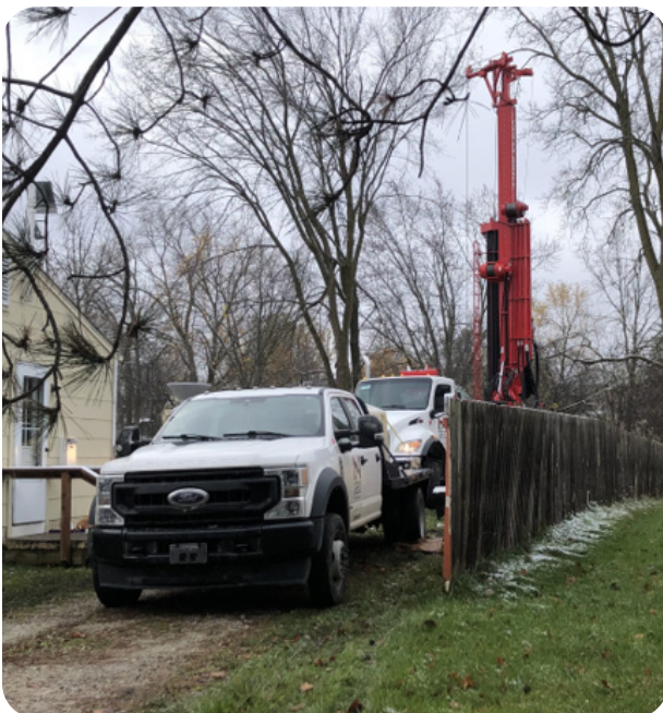
Geothermal rig at the Bryant Community Center drilling the vertical wells for the Center's geothermal heating and cooling system.
